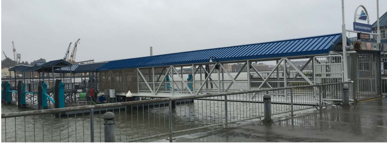
Figure 59: Passenger ferry dock at Vallejo. The ticket office and lobby is in the building in the far right background.
