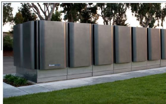
Figure 8: Bloom Energy ES-5700 solid oxide fuel cells, each producing power at 210 kW each. Photo from Reference [43].
