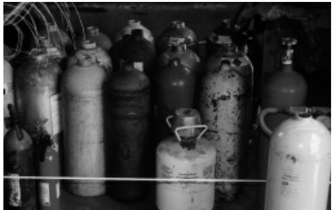
Compressed air tanks improperly tested by Fire Service, Inc.
