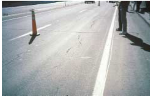
Figure 4.79: AC Low Severity Fatigue Type Cracking
