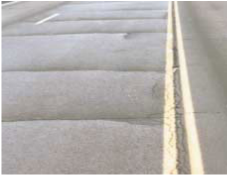
Figure 4.94: High Severity AC/Composite Reflection Cracking
