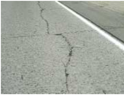
Figure 4.89: JCP High Severity Longitudinal Cracking
