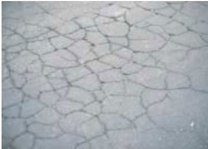
Figure 4.78: AC Chicken Wire/Alligator Fatigue Type Cracking in Wheel path
