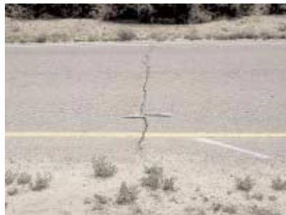
Figure 4.97: High Severity AC Transverse Cracking
