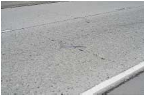
Figure 4.92: JCP High Severity Transverse Cracking
