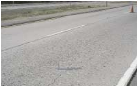
Figure 4.87: JCP Low Severity Longitudinal Cracking
