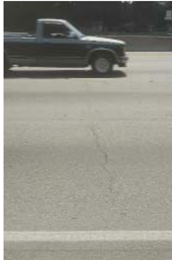
Figure 4.95: Low Severity AC Transverse Cracking
