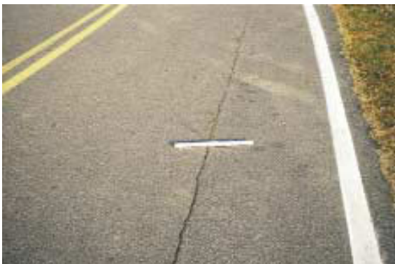
Figure 4.77: AC Moderate Severity Longitudinal Cracking (Wheel path)
