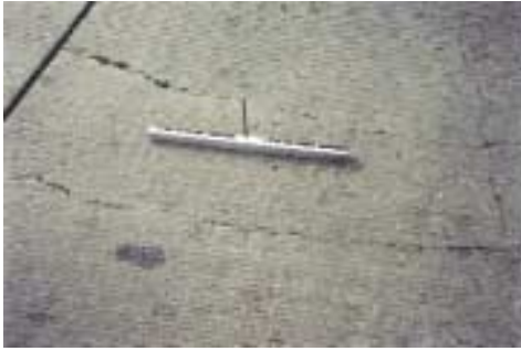
Figure 4.83: Low Severity CRCP Punchout Cracking
