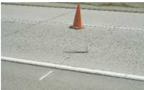
Figure 4.91: JCP Moderate Severity Transverse Cracking
