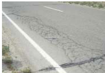
Figure 4.81: AC High Severity Fatigue Type Cracking
