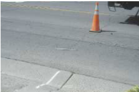
Figure 4.96: Moderate Severity AC Transverse Cracking
