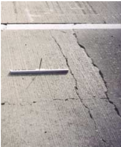
Figure 4.84: Moderate Severity CRCP Punchout Cracking
