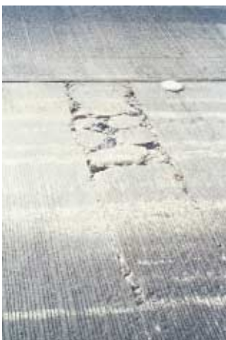
Figure 4.85: High Severity CRCP Punchout Cracking
