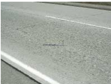
Figure 4.88: JCP Moderate Severity Longitudinal Cracking
