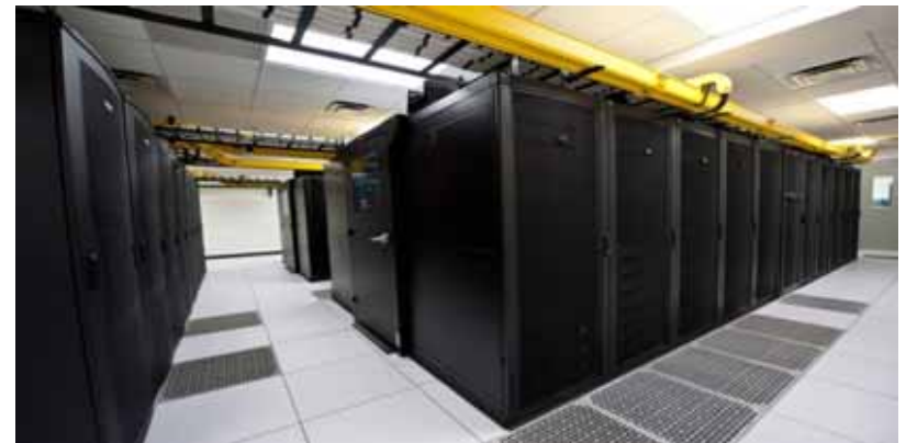
NREL Data Center storage arrays
