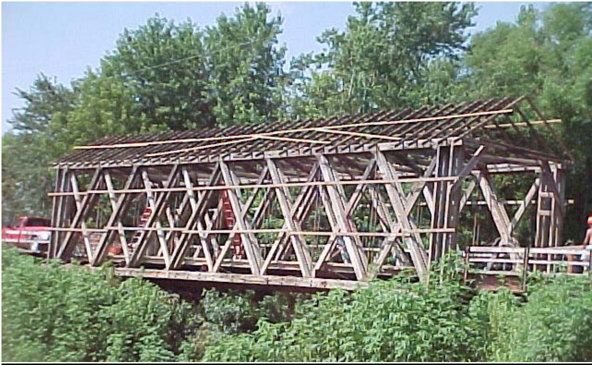
Figure 37 The timber and metal Howe truss system is easy to see with the siding removed. Note the rafters have no ridge board.
