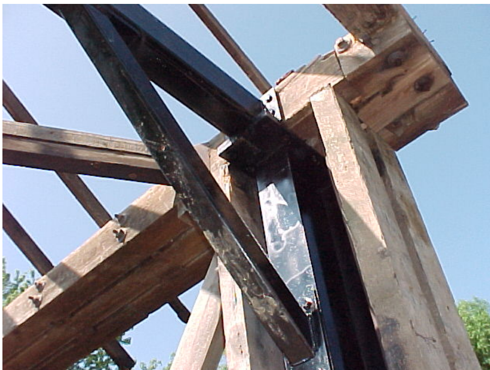
Figure 26 Juncture of the steel portal upright and beam, as bolted to the wooden bridge.
