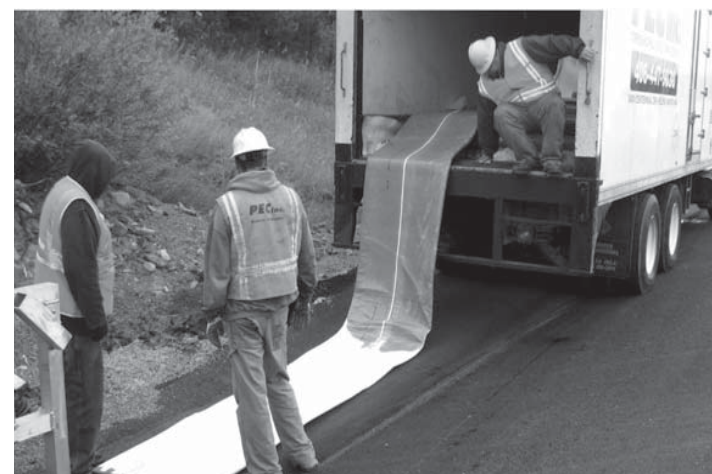
A new pipe installed inside the existing culvert eliminated the need for roadway excavation and traffic disruption.
