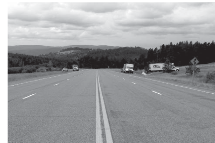
Because the work was done beyond the roadway shoulders, the Montana culvert project did not affect U.S. 12 travelers.
