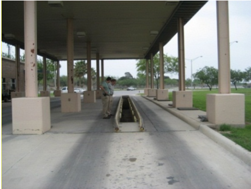
Above: Rio Grande City, TX. This inspection pit is typical for what is planned for each border facility inspection lane.
