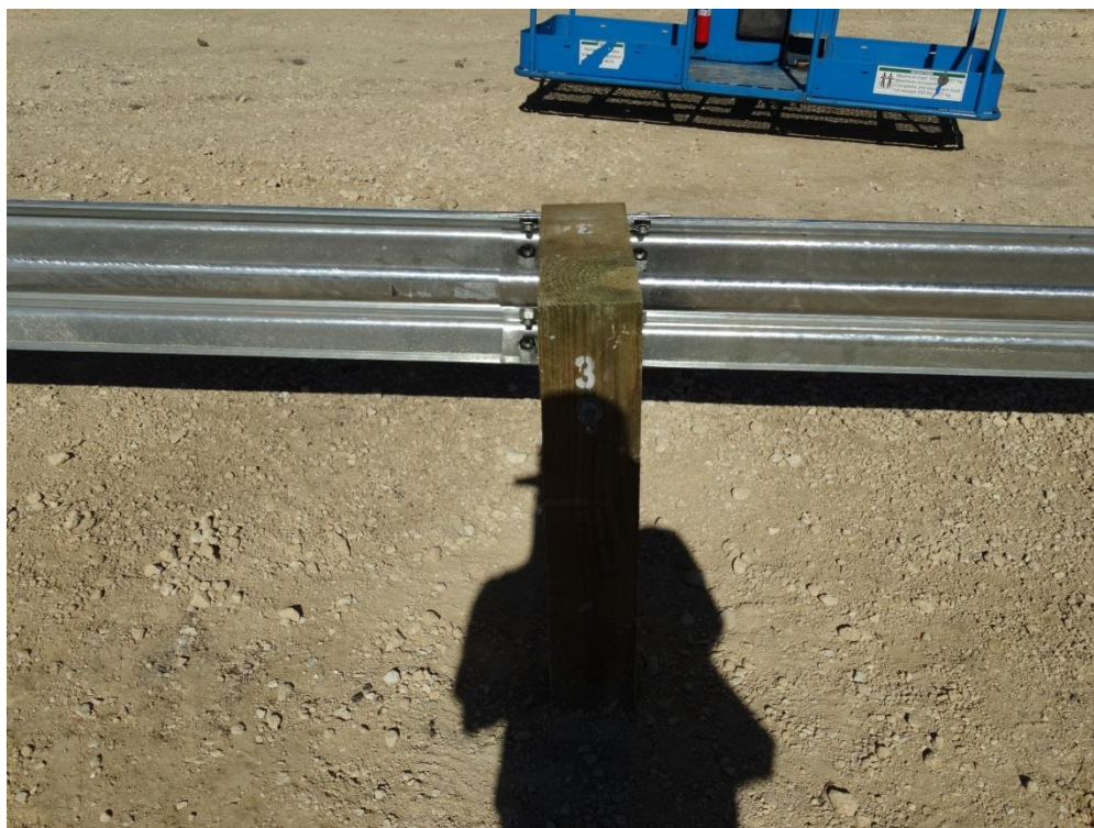
Figure 2.12: First Guardrail Panel Splice Joint – Non-Traffic Side (Nuts Painted for Visibility in Video)
