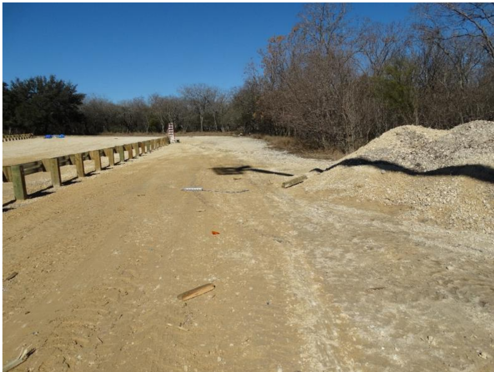
Figure 3.51: Post Test – Debris Field on Non-Traffic Side
