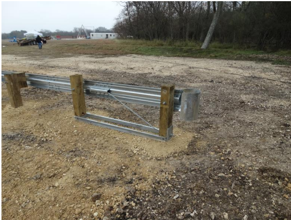
Figure 2.19: Downstream Anchor Terminal at Posts 26 and 27 – Non-Traffic Side
