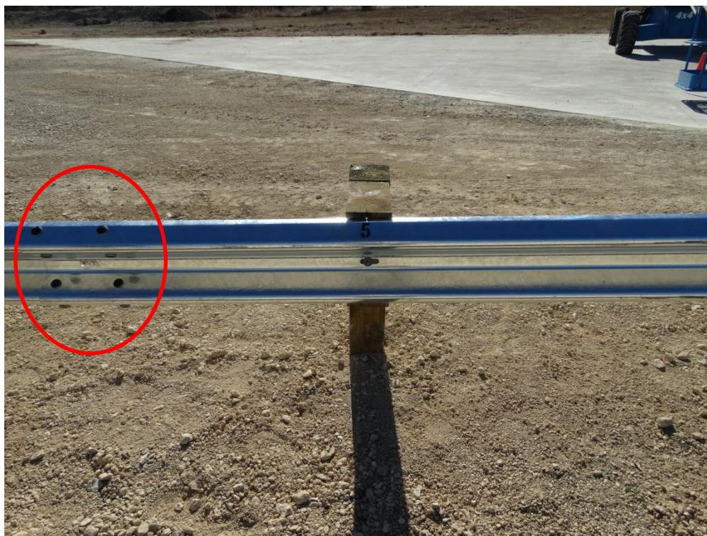
Figure 2.13: Second Guardrail Panel Splice Joint Mid-Span between Posts 5 & 6 – Traffic Side (Splice Bolts Painted for Visibility in Video)
