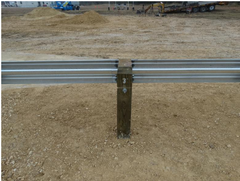
Figure 2.12: First Guardrail Panel Splice Joint – Back Side (Nuts Painted for Visibility in Video)
