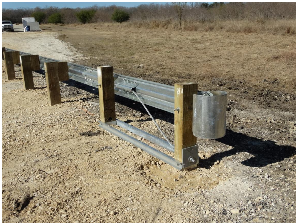
Figure 2.20: Downstream Anchor Terminal at Posts 26 and 27 – Non-Traffic Side
