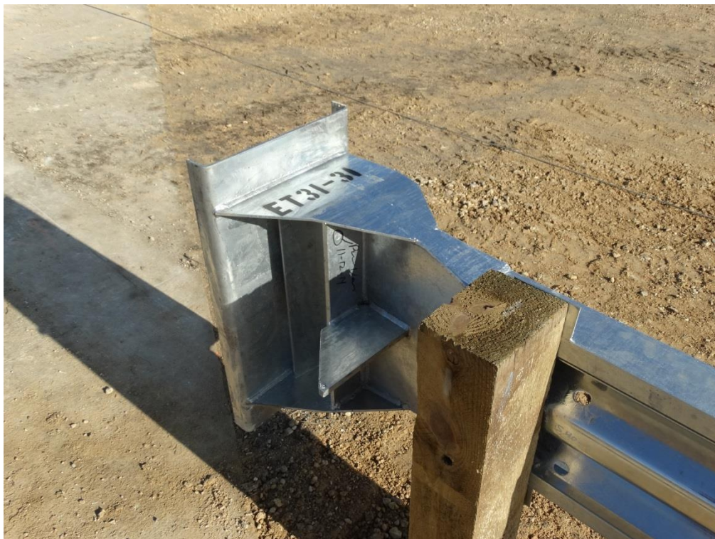
Figure 2.18: ET Plus Head Looking Upstream at Post 1 (see Appendix B for Dimensions)
