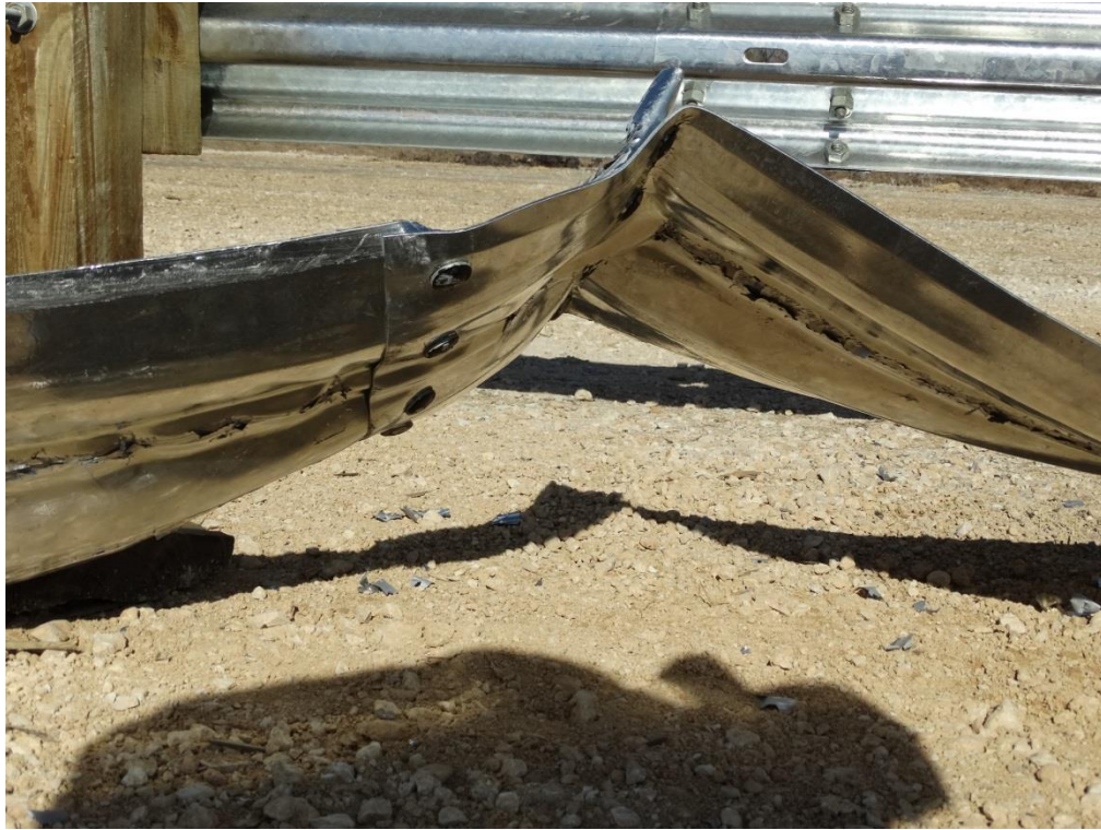
Figure 3.24: Post Test – Extruded Guardrail Splice from between Posts 5 & 6 (Splice Bolts Painted Pre-Test for Visibility in Video)
