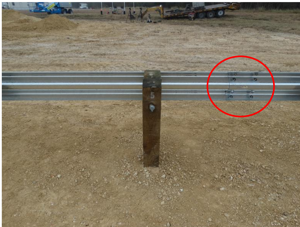
Figure 2.14: Second Guardrail Panel Splice Joint Mid-Span between Posts 5 & 6 – Back Side (Nuts Painted for Visibility in Video)
