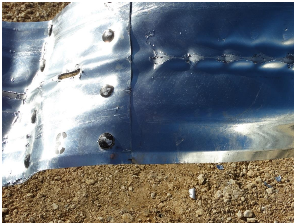
Figure 3.22: Post Test – Extruded Guardrail Splice from Post 3 (Splice Bolts Painted Pre-Test for Visibility in Video)
