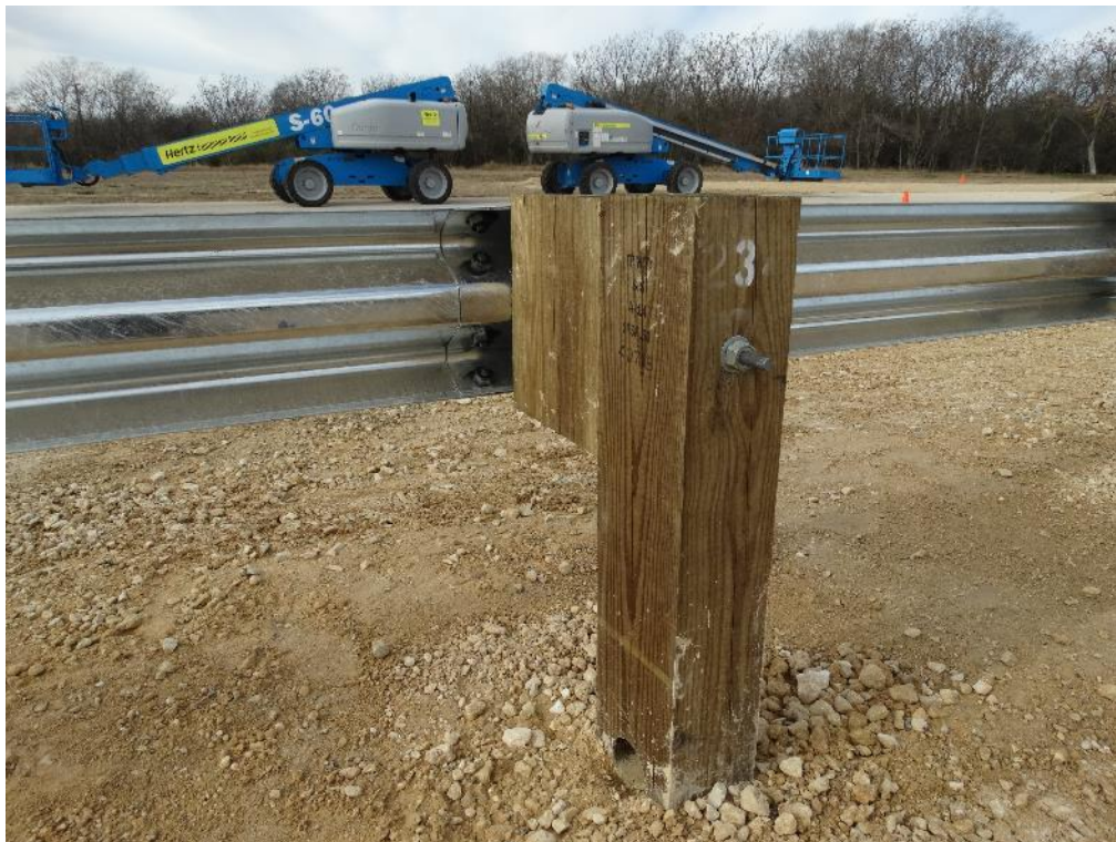
Figure 2.12: First Guardrail Panel Splice Joint – Non-Traffic Side (Nuts Painted for Visibility in Video)
