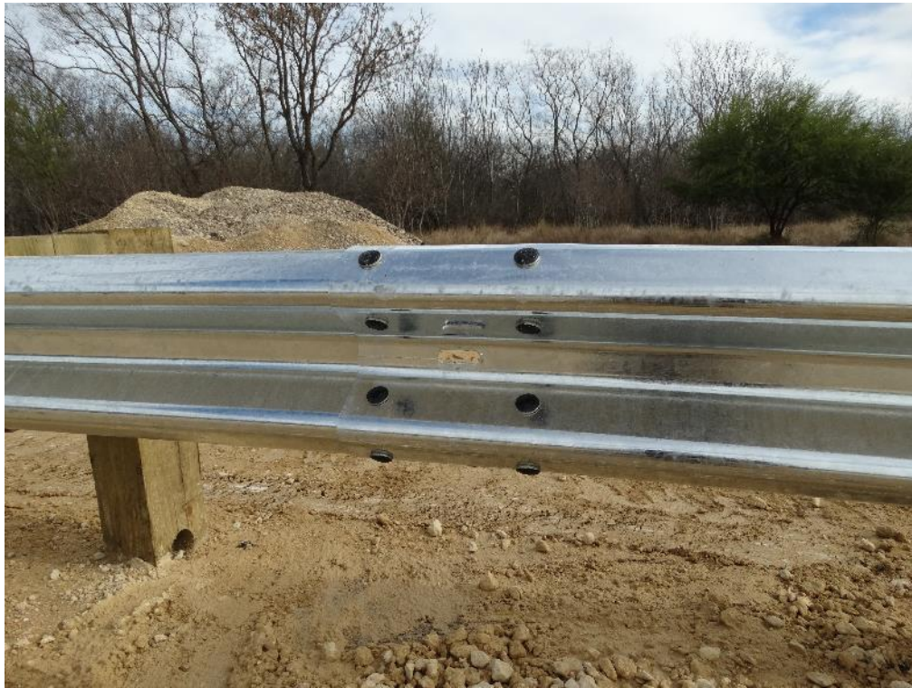
Figure 2.13: Second Guardrail Panel Splice Joint Mid-Span between Posts 5 & 6 – Traffic Side (Splice Bolts Painted for Visibility in Video)
