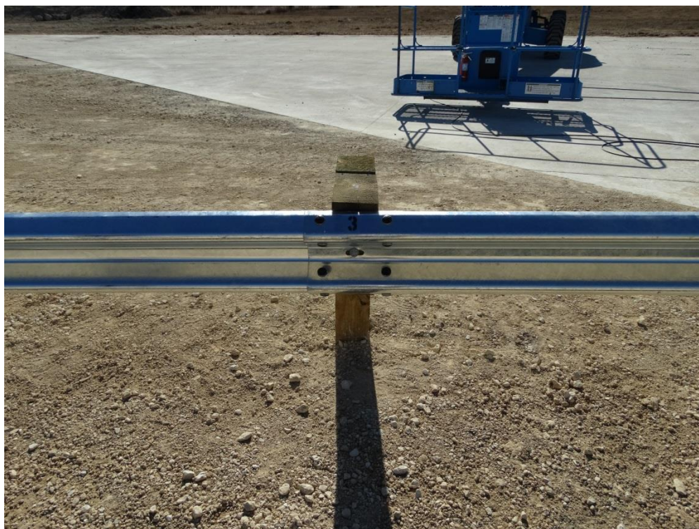
Figure 2.11: First Guardrail Panel Splice Joint – Traffic Side (Splice Bolts Painted for Visibility in Video)
