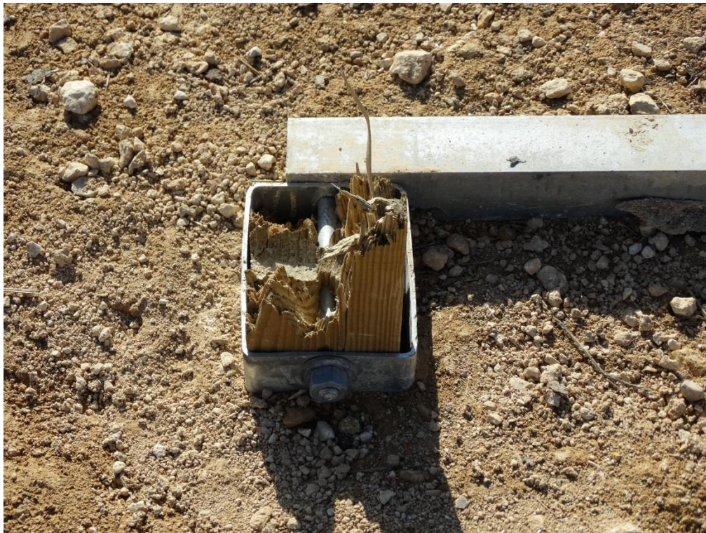
Figure 3.9: Post Test – Post 2 Foundation Sleeve
