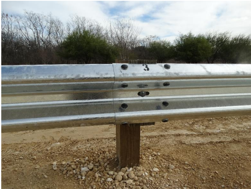
Figure 2.11: First Guardrail Panel Splice Joint – Traffic Side (Splice Bolts Painted for Visibility in Video)
