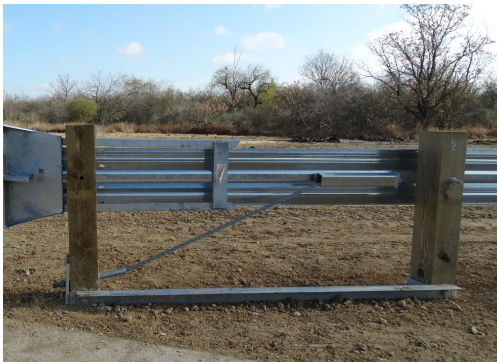
Figure 2.8: ET Plus Head and Anchor Cable Assembly
