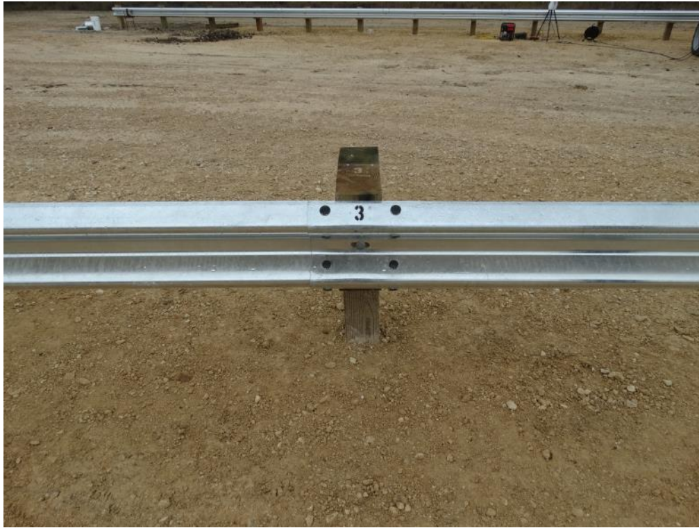
Figure 2.11: First Guardrail Panel Splice Joint – Traffic Side (Splice Bolts Painted for Visibility in Video)
