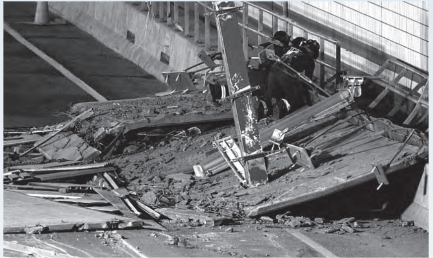
Boston, MA — Collapsed section of the I-90 eastbound tunnel. Photo by Matthew West, Boston Herald.
