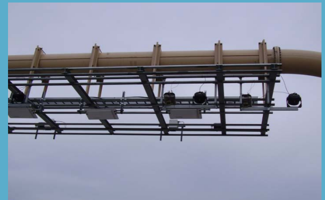
Electronic Tolling Equipment
