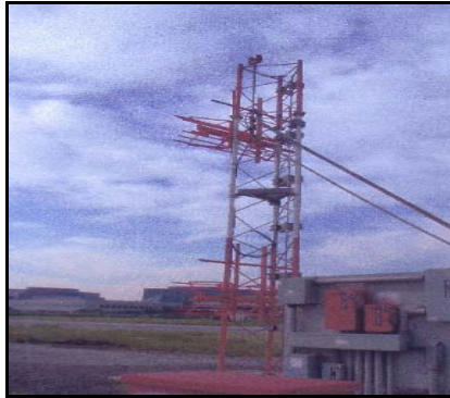
Figure 8. Glide Slope Antenna at Long Beach Airport
