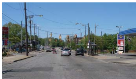
RSA finding: Degraded Pavement Markings
