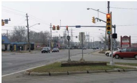
RSA finding: Conflicting Traffic Signal Indications
