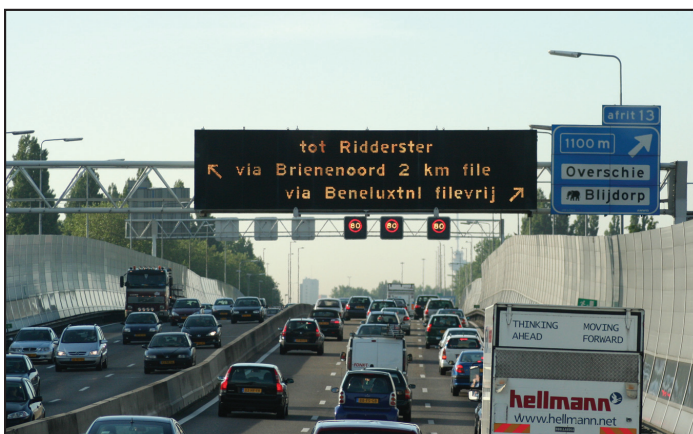
Dynamic Route Information Panels (DRIPs) in Netherlands. Source: Robert Hull
