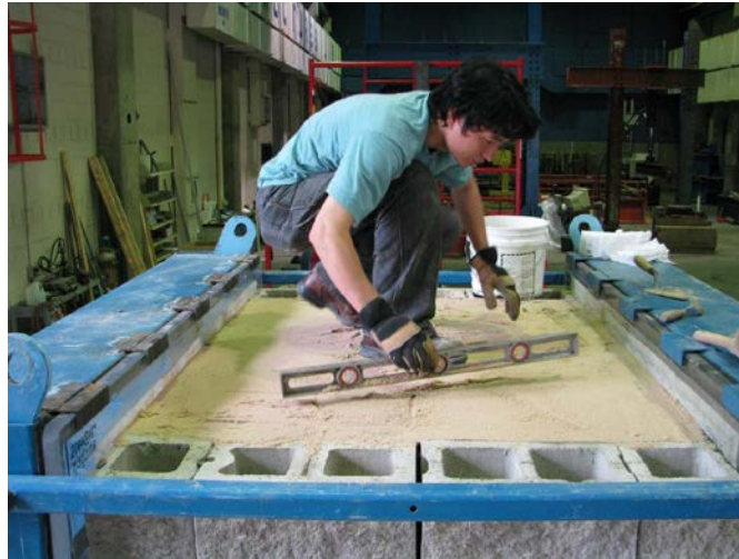
Figure 131. Photo. Completion of compaction of the composite mass and leveling the top surface with 0.2-inch (5-mm)-thick sand layer.
