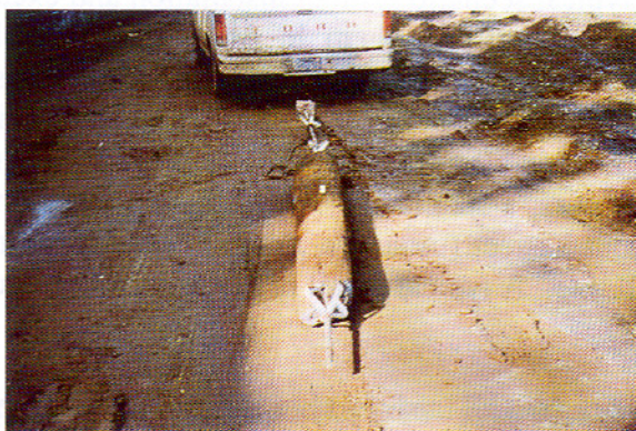
P50. Exhumed sacrificial test nail. Note lack of grout from bottom centralizer to tip of nail. Problem resulted from (1) not placing tremie grout pipe completely to bottom of drillhole; and (2) using too stiff a grout (e.g., shotcrete mix).
