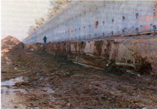
P46. Mass excavation stopped short of final wall line to leave a stabilizing (buffer) berm.
