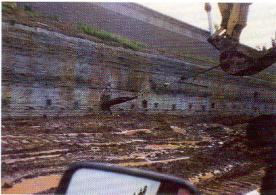
P49. Exhuming failed sacrificial test nail.
