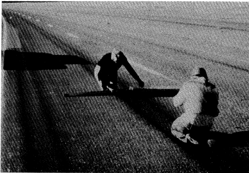
Figure 14. An example of rutting.
