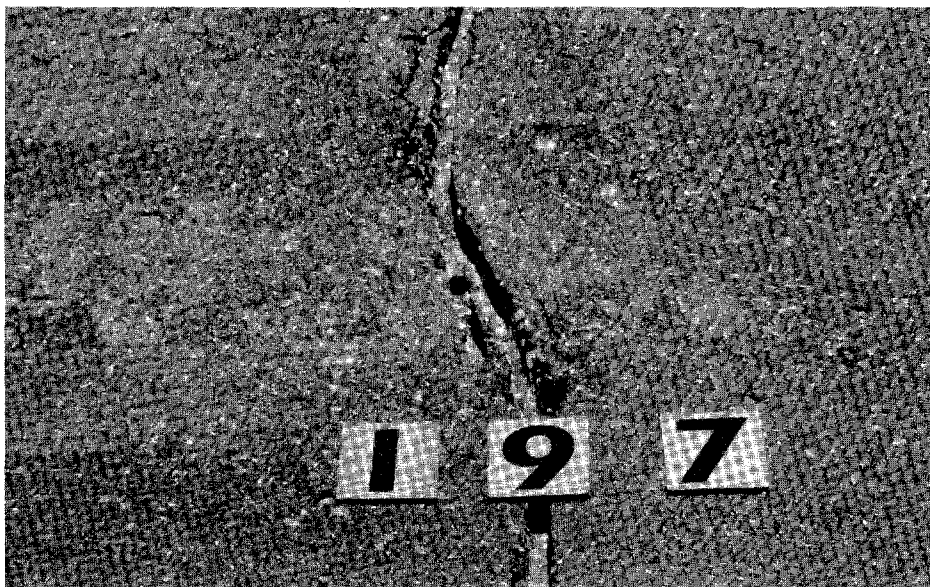
Figure 5-6. Crack segment missed by cutting equipment.
