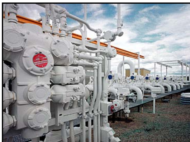
Figure 4. Piping at Facility Pump Station
