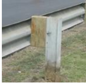
Figure 41. Photo. Barrier type 15—W-beam strong post. (14)
