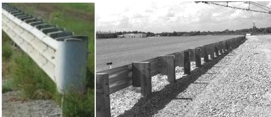
Figure 14. Photo. Case No. 2005012696122 post-crash Thrie beam strong post (left) contrasted with comparative catalog image (right). (4,16)
