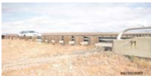
Figure 56. Photo. Barrier end treatment type 10—W-beam terminal connector shoe. (14)
