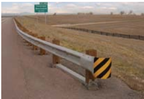
Figure 54. Photo. Barrier end treatment type 7—terminal end sections (boxing glove). (14)
