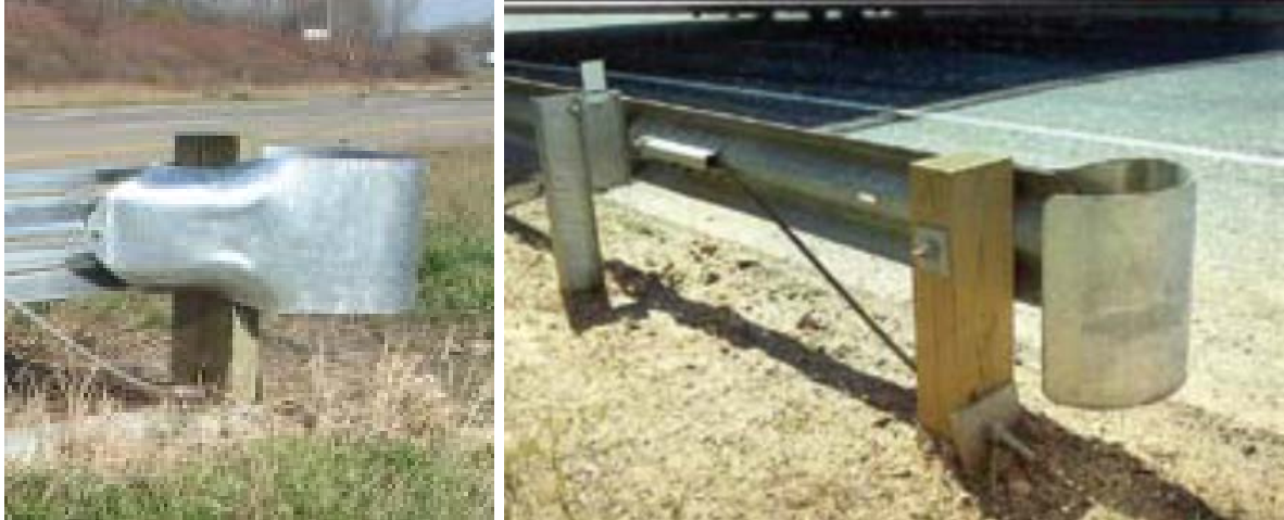
Figure 15. Photo. Case No. 2005012696122 post-crash Thrie beam strong post (left) highlighting non-energy absorbing slotted rail terminal contrasted with comparative catalog image (right). (4,14)
