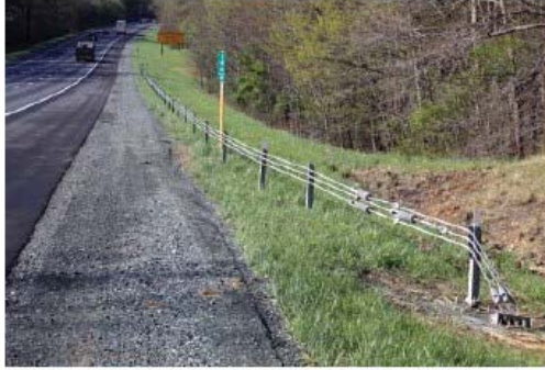
Figure 35. Photo. Barrier type 9—low-tension cable guardrail. (21)
