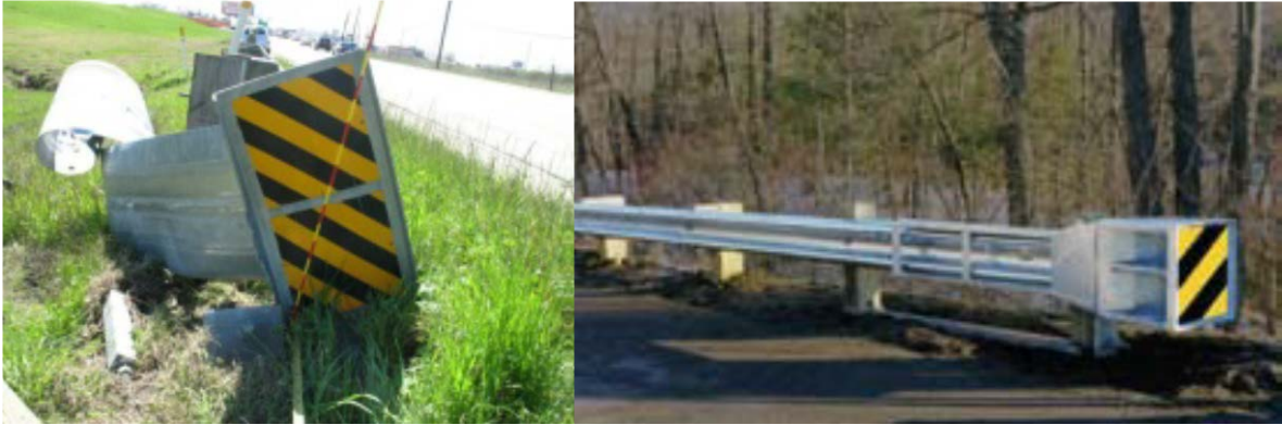
Figure 12. Photo. Case No. 2005049602183 post-crash W-beam strong post highlighting energy absorbing end treatment. (4,14)
