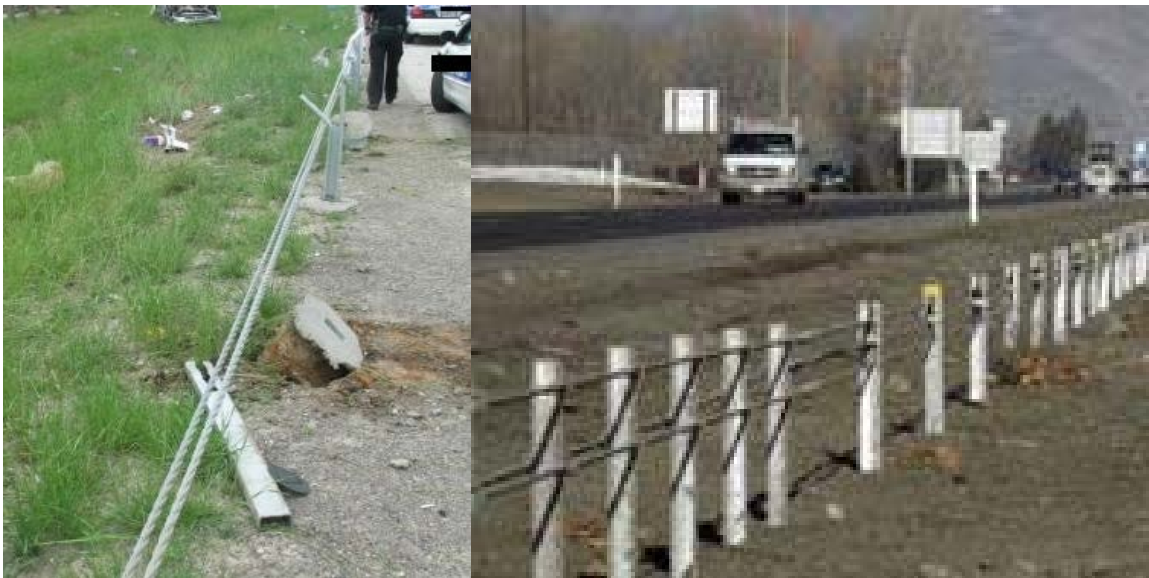
Figure 13. Photo. Case No. 2005049602403 post-crash high-tension cable guardrail systems (left) contrasted with comparative catalog image (right). (4,15)
