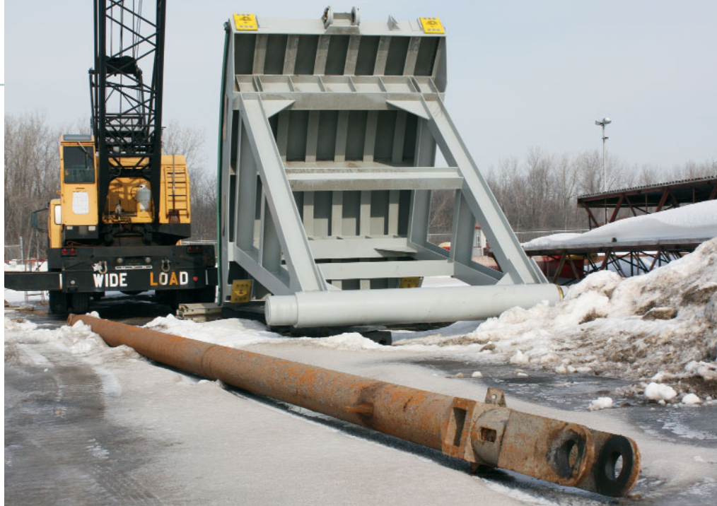
RIGHT: Preparing for installation of a new single skin culvert valve at the upstream south side of Snell Lock.
