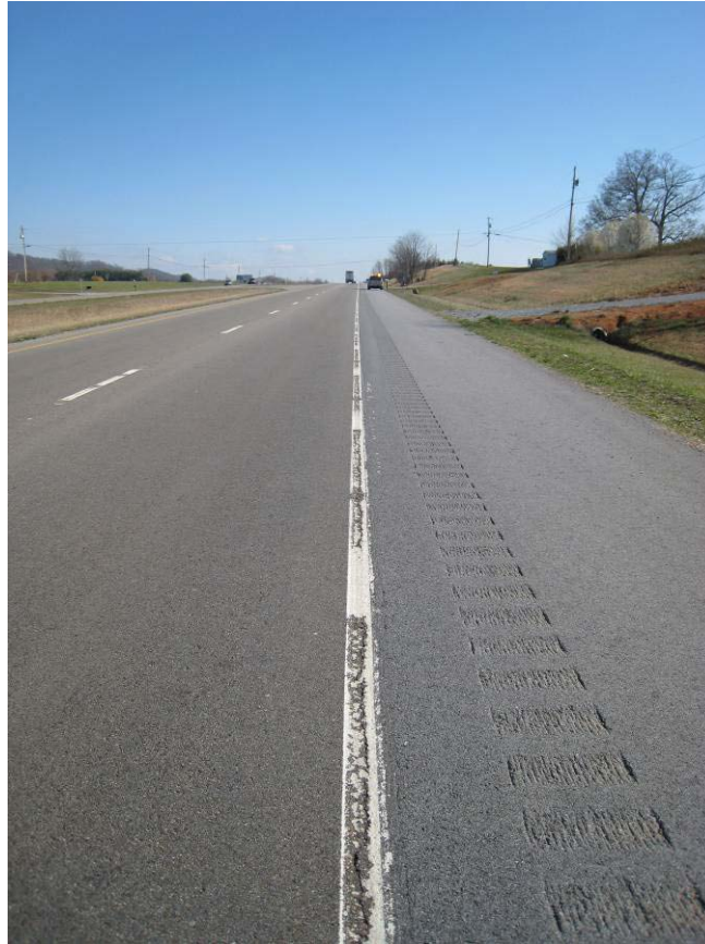
Figure 8. Photo. Tusculum, TN, test deck section 1 TN-T presence failure.
