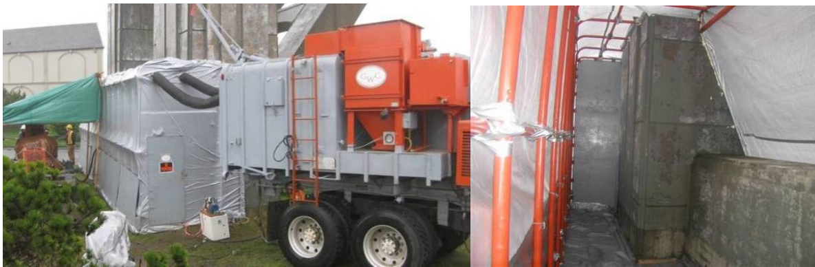
Figure 4.31: Containment enclosure with negative pressure system and blast pot assembly: (left) external view; (right) internal view.
