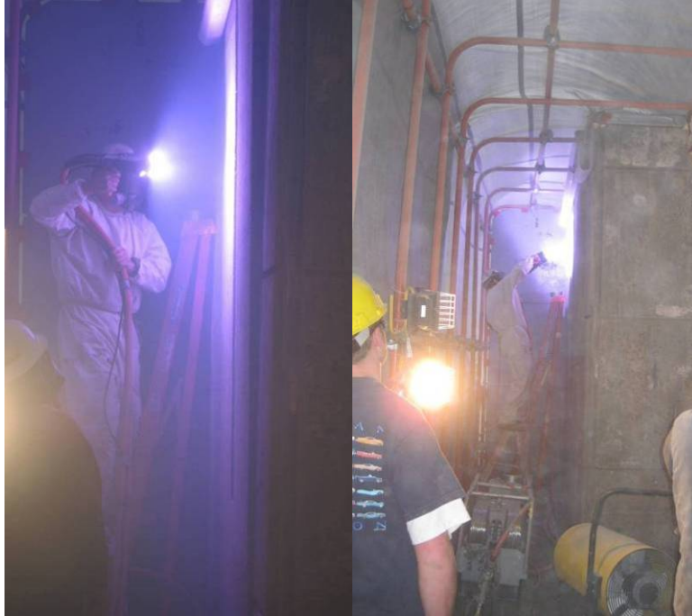
Figure 4.37: GWC worker applying new anode to the south face of the west pier.
