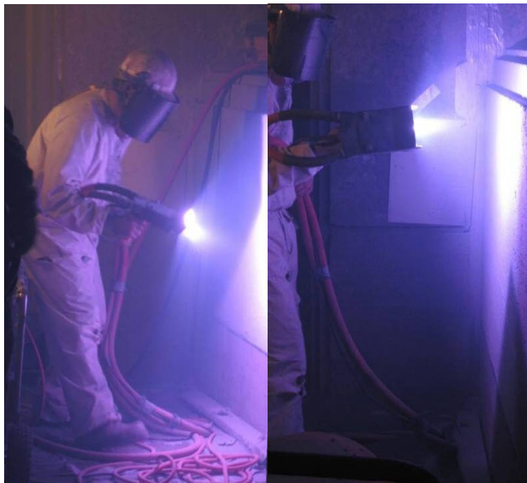
Figure 4.38: GWC worker applying new anode to the pile cap section of pier structure.
