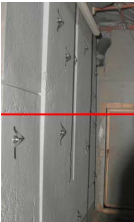
Figure 4.41: South face of the east pier divided into two sections, high and low sand content. Low sand content section is below the red line in the picture.
