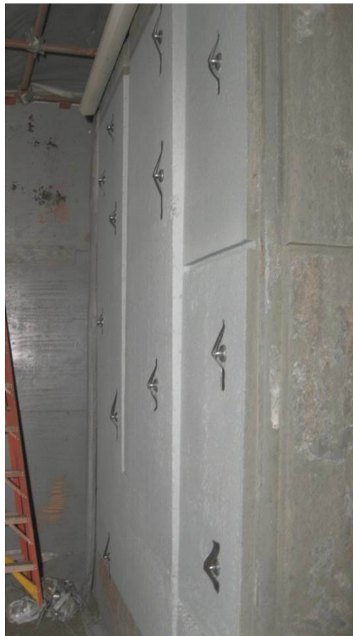
Figure 4.39: South face of the west pier profiled with a #8 nozzle and high sand, control section.
