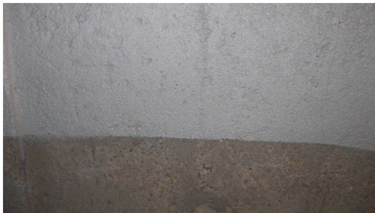
Figure 4.36: Irregular concrete surface due to paste loss.
