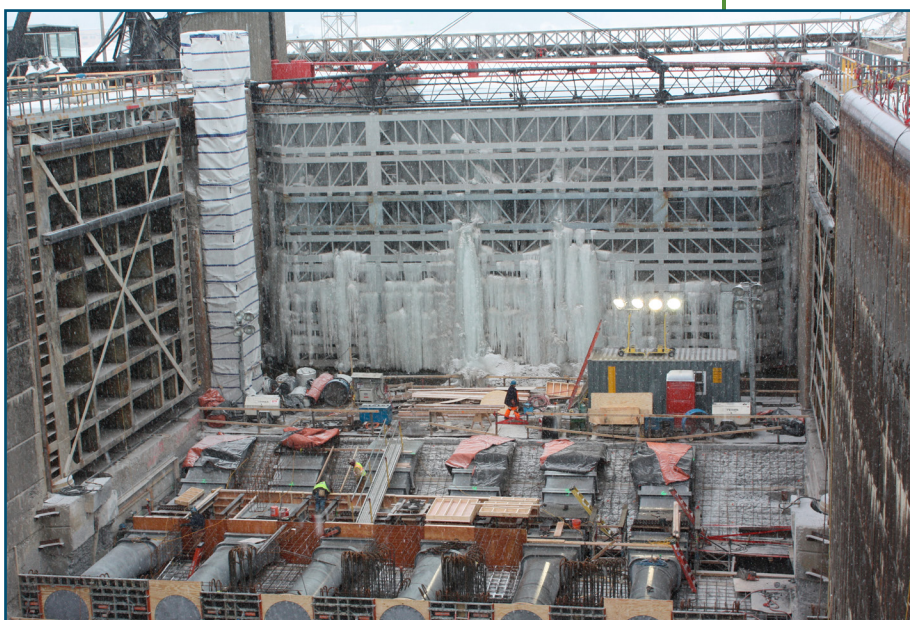
Installation of the new ice flushing system at Snell Lock, Massena, New York.
