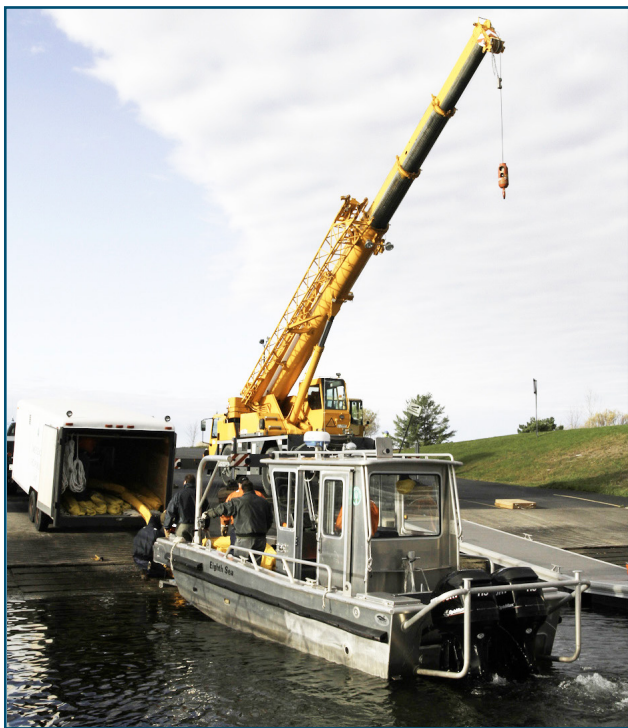
SLSDC personnel prepare to deploy boom as part of an on-the-water exercise during the Emergency Preparedness Committee on Civil Transportation workshop.
