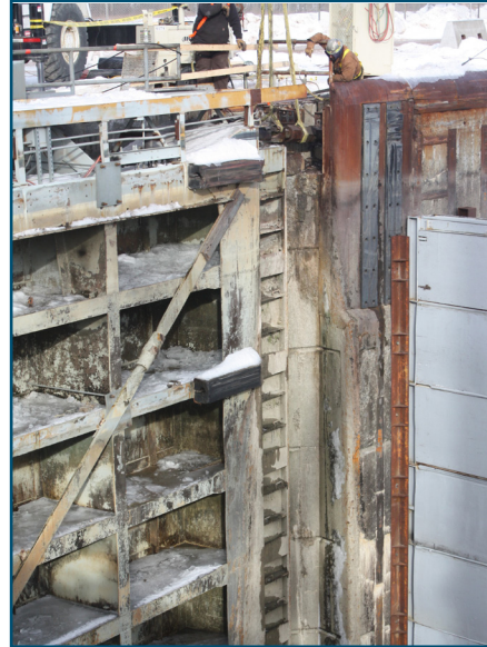
Contractor is working on the downstream north miter gate leaf at Eisenhower Lock.
