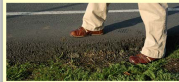
View of southeast corner at intersection of Indian Road. Photo shows substantial pavement edge drop near turning radius.
