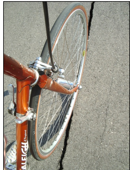
Figure 22: Cracking can cause trip hazards as well as hazards for bicyclists and wheelchair users. This crack is on a shared use path.
