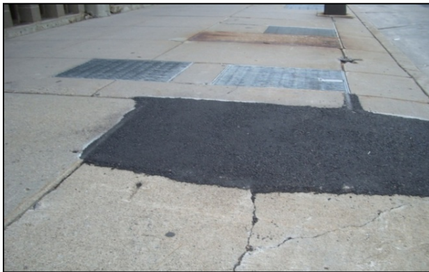
Figure 23: Wedge has been placed to mitigate the hazard caused by a raised sidewalk slab. Note the extensive and appropriate ramping of the wedge.
