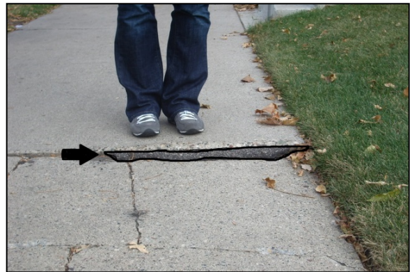
Figure 24: A small wedge may still create a hazard or be difficult to navigate in a wheelchair. This wedge had deteriorated over time.
