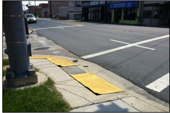
Figure 10: Damaged detectable warning fields.
