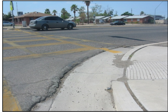
Figure 14: Asphalt pushed up against curb ramp. Photo by Tom Fisher
