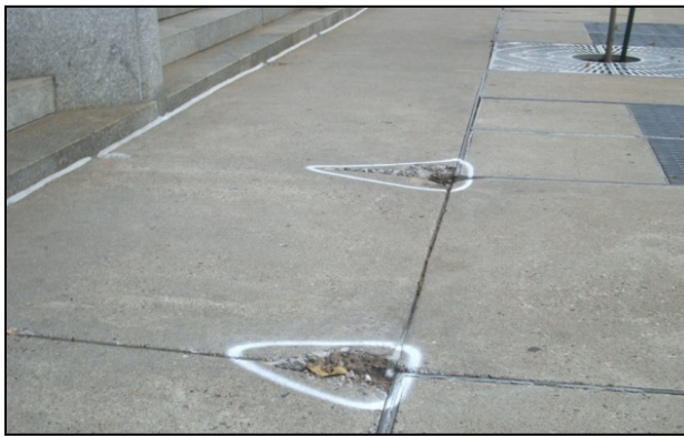
Figure 20: Missing areas of concrete have been marked for repair.
