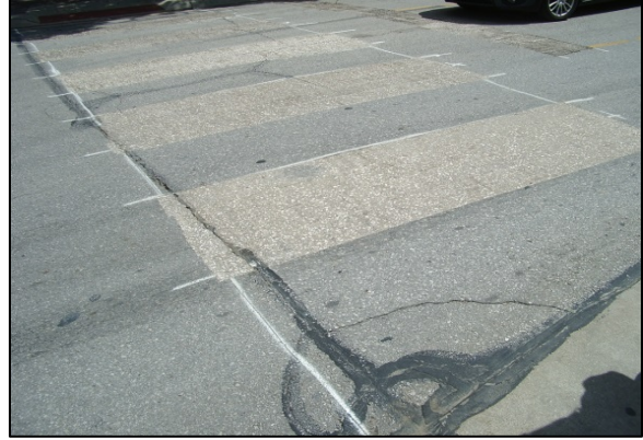
Figure 11: A street is prepared for the installation of new crosswalk in-laid markings.
