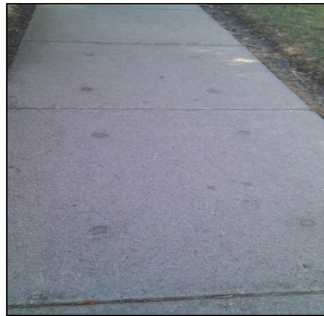
Figure 28: These panels were mud-jacked more than 20 years ago and are still in good condition so if done properly this can be a permanent fix.
