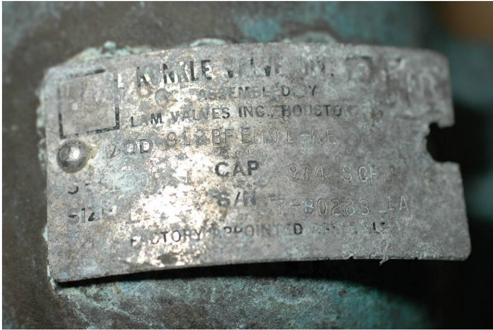
Figure 23: Shows PRD identified as 08H127-2
