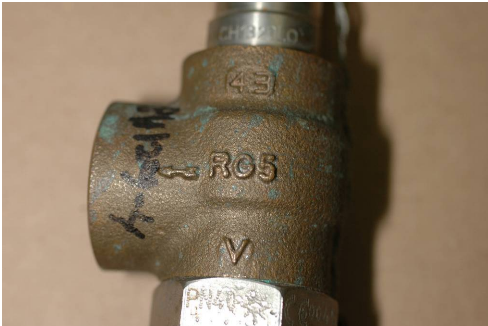
Figure 58: Shows PRD identified as 08H127-4
