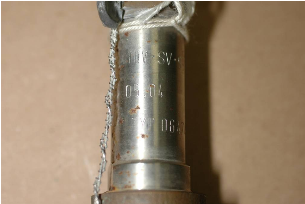
Figure 60: Shows PRD identified as 08H127-4
