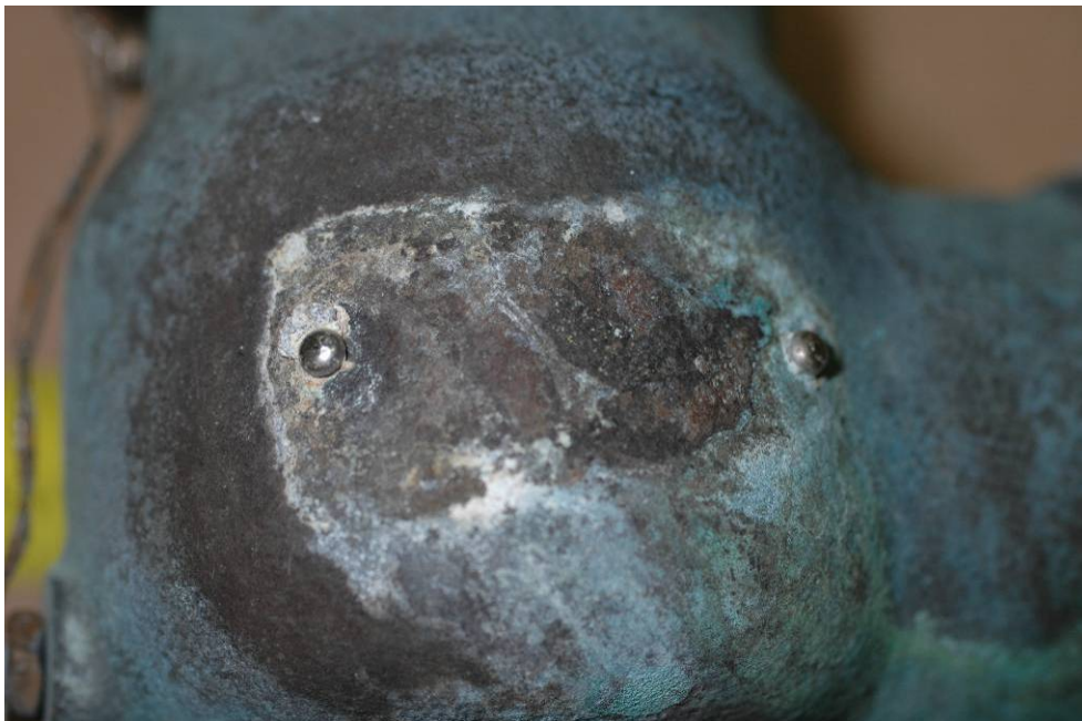
Figure 34: Shows PRD identified as 08H127-3
