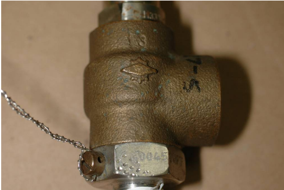
Figure 71: Shows PRD identified as 08H127-5
