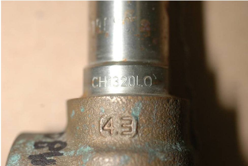
Figure 61: Shows PRD identified as 08H127-4
