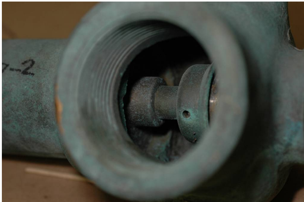
Figure 20: Shows PRD identified as 08H127-2
