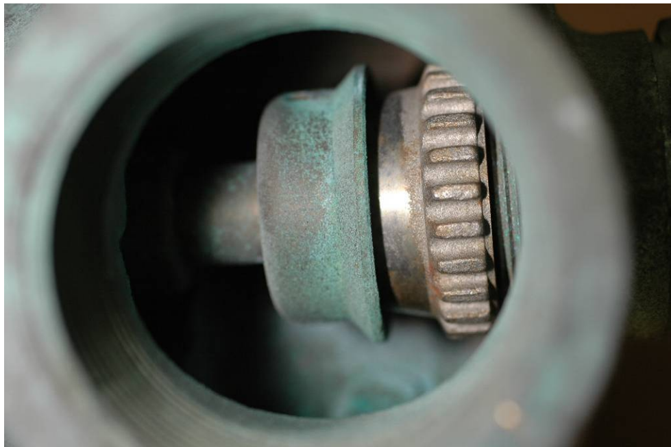
Figure 8: Shows PRD identified as 08H127-1
