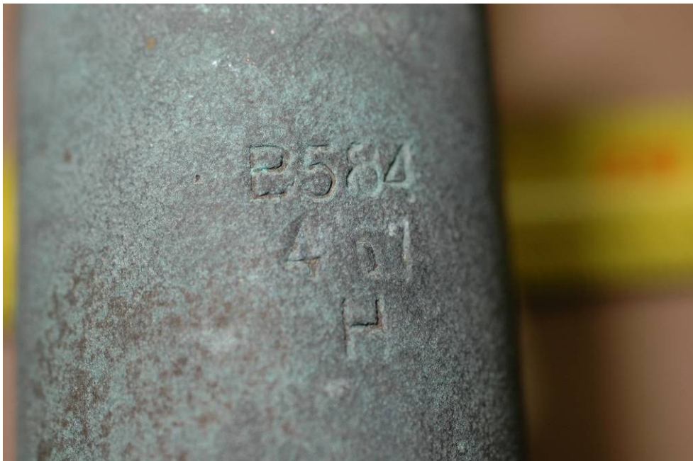
Figure 22: Shows PRD identified as 08H127-2
