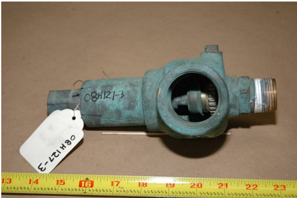
Figure 30: Shows PRD identified as 08H127-3
