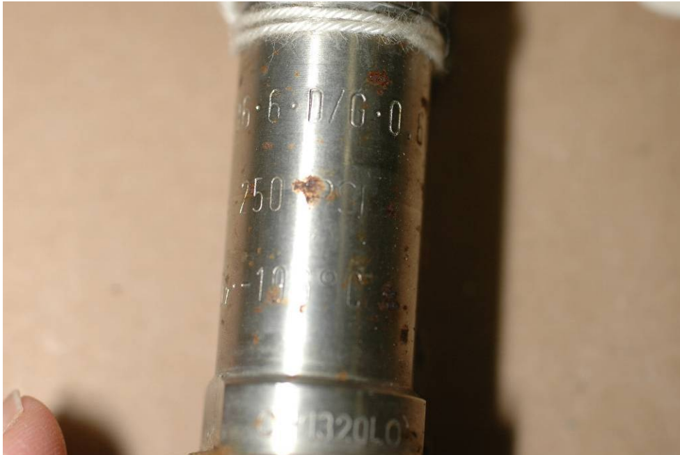
Figure 59: Shows PRD identified as 08H127-4
