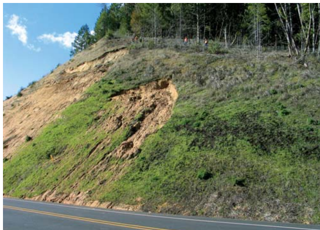
Figure 2 ~ This debris slide took place two years after construction, when grasses were fully established. To preclude these kinds of problems, revegetation should have the establishment of long-term plant communities, not just quick cover, as a goal.
