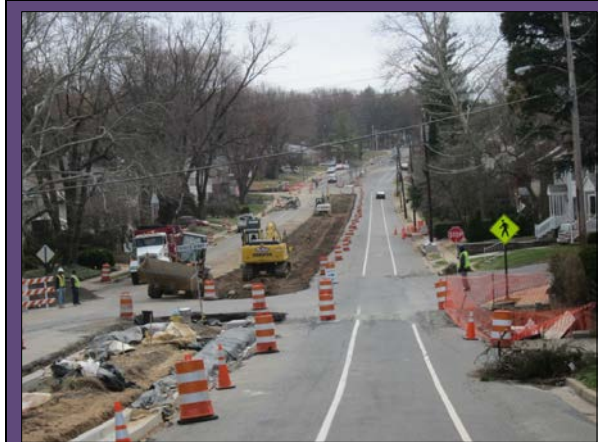
Photograph of roadway under construction for a green streets project in Arlington, Virginia. Project includes pedestrian intersection improvements and the creation of a bio-retention swale in the median. This project is part of the county's Neighborhood Conservation Program which directly engages citizens in identifying project scope and needs within their neighborhoods and prioritizing projects annually.
