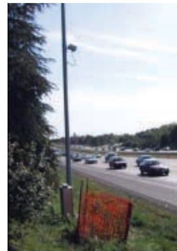
Remote Traffic Microwave Sensor (RTMS)
