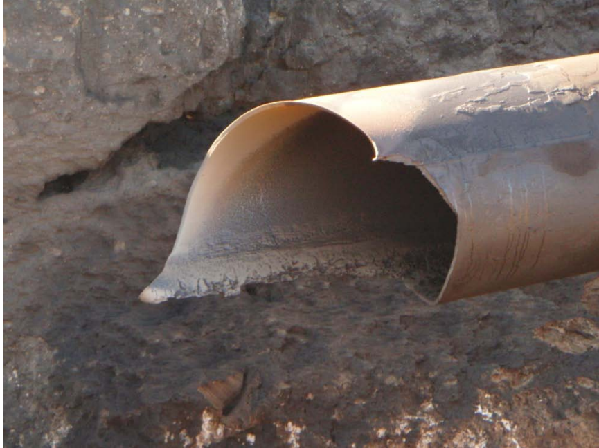
Figure D3 – End of Rupture Location
