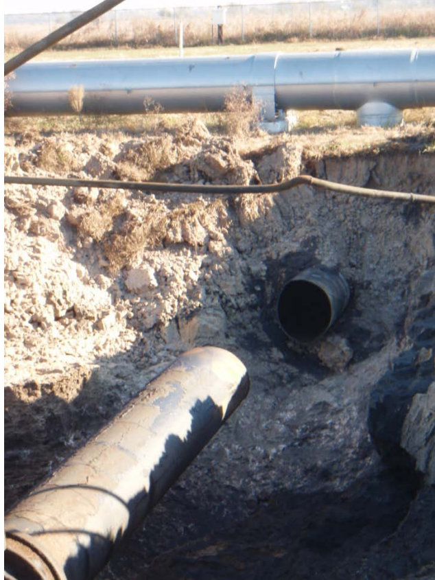
Figure D1 - Rupture Location
