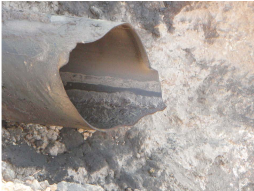
Figure D2 – End of Rupture Location
