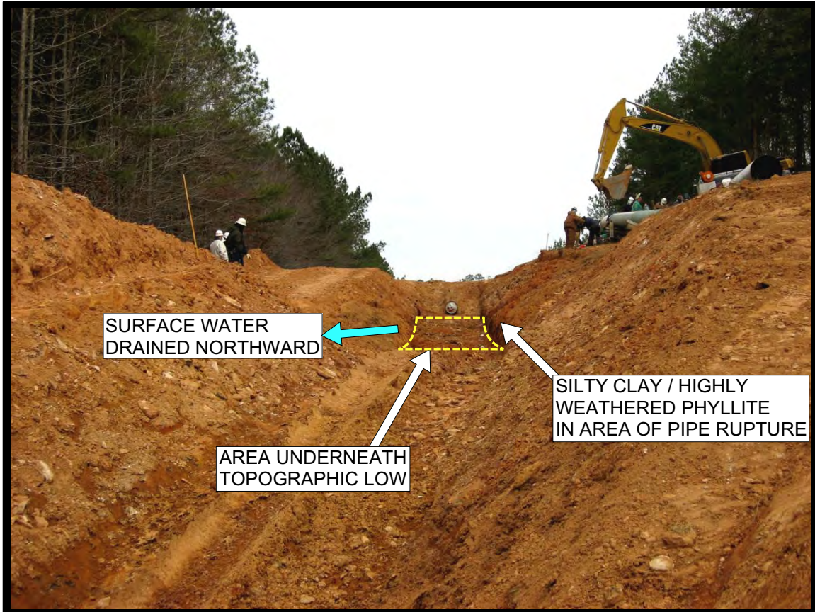
PHOTOGRAPH 2. AREA OF PIPE FAILURE (VIEW IS TOWARD EAST)
