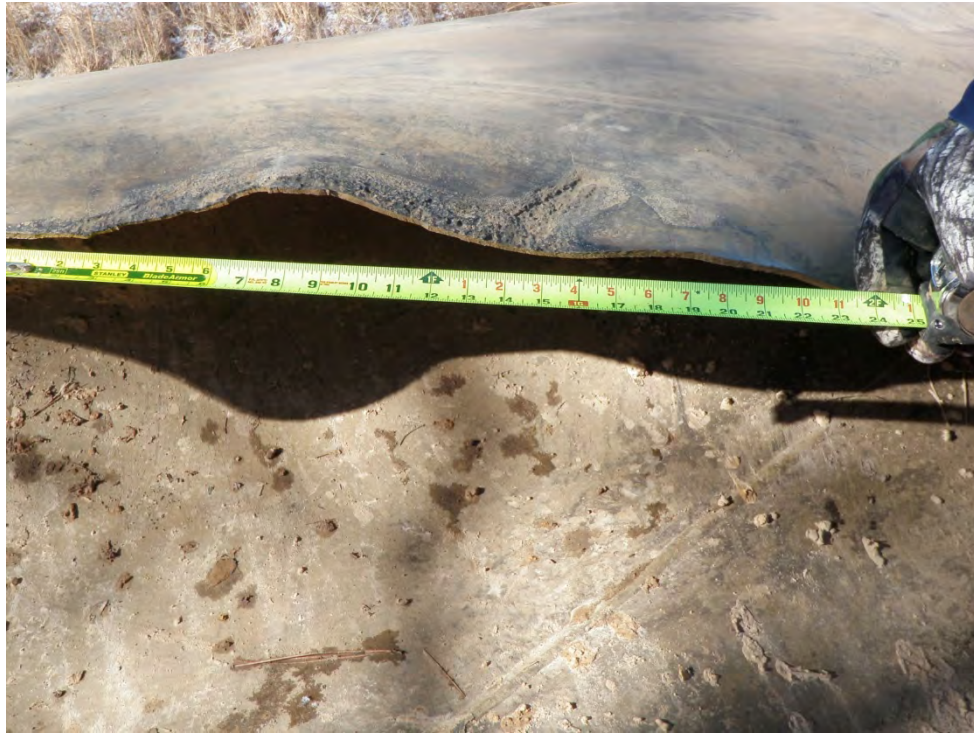
Corrosion pitting in a section of expelled pipe
