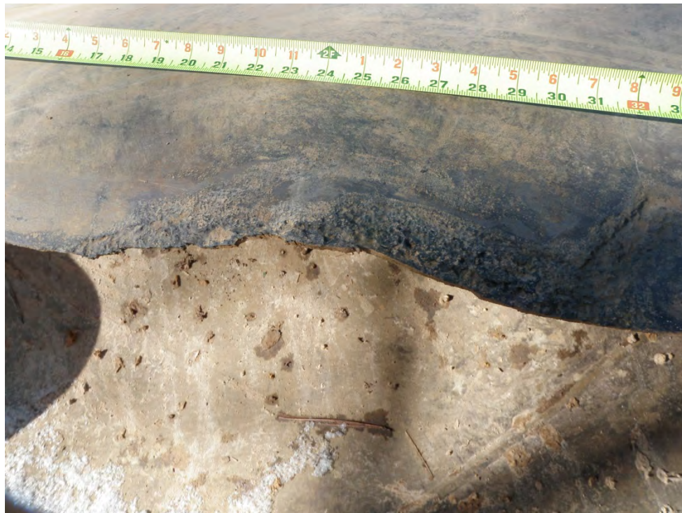
Corrosion pitting, same pipe section (zoomed-in)
