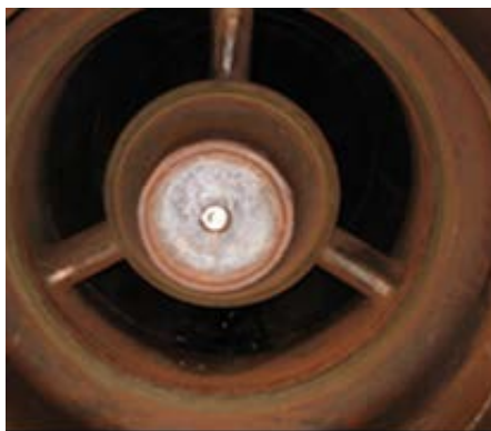
Figure 2 - Check Valve Center with sheared bolt
