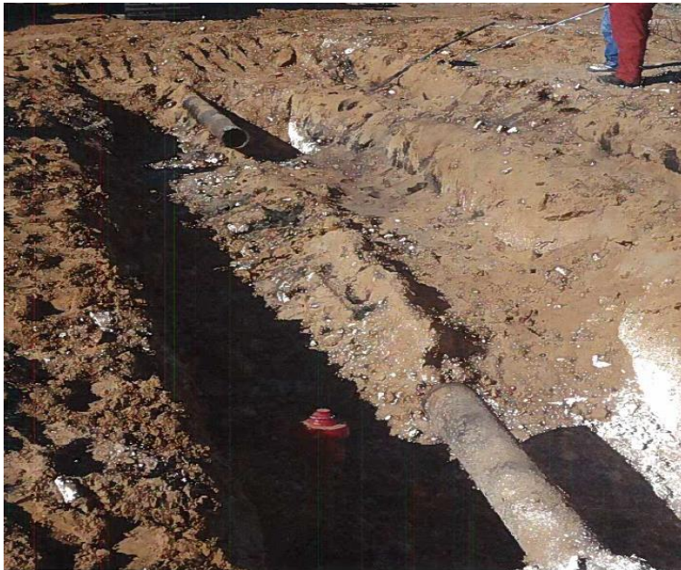
Site After Flash Fire
