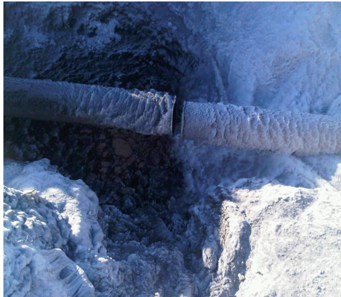
Failed Girth Weld
