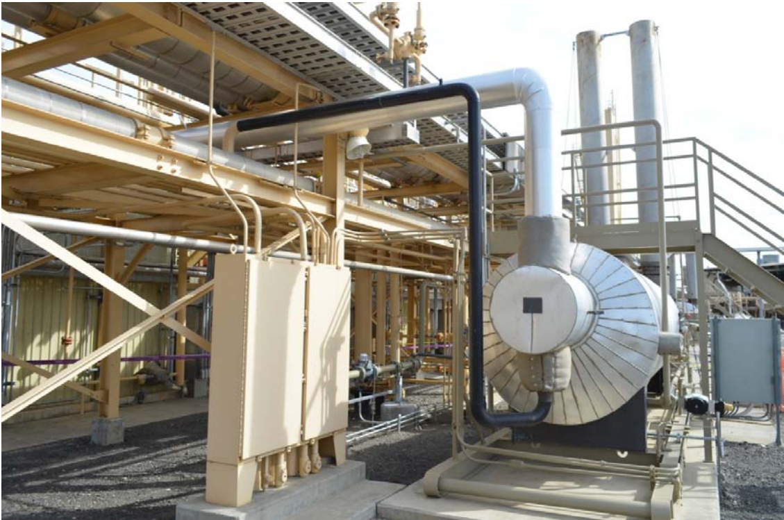
The LNG-2 Salt Bath Heater which was identical to the LNG-1 Salt Bath Heater. The 4-inch inlet gas piping is painted black.
