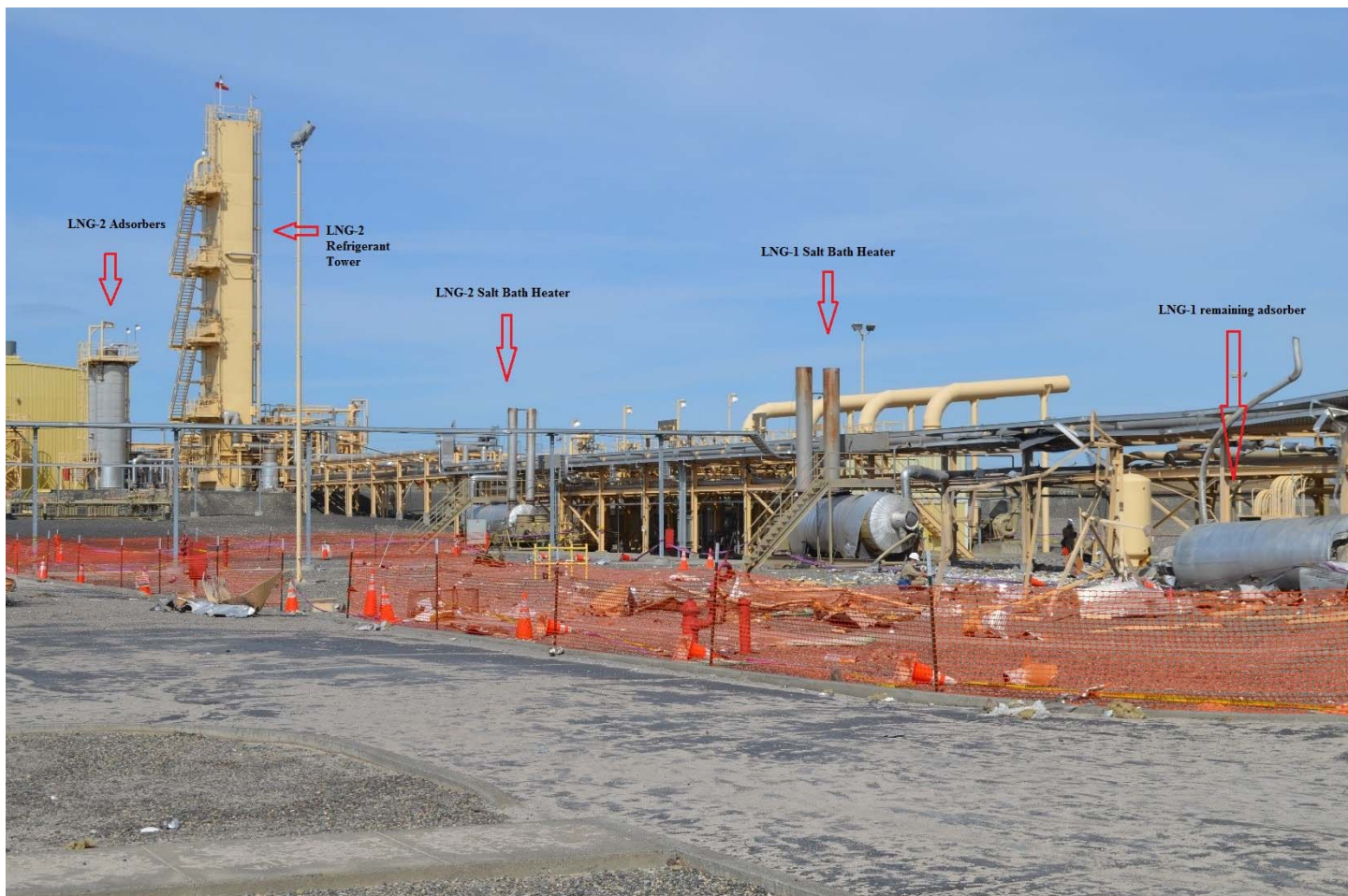
LNG-1 and LNG-2 purification systems. Looking northeast. Undamaged LNG-2 adsorbers, refrigerant tower and Salt Bath Heater center left.
