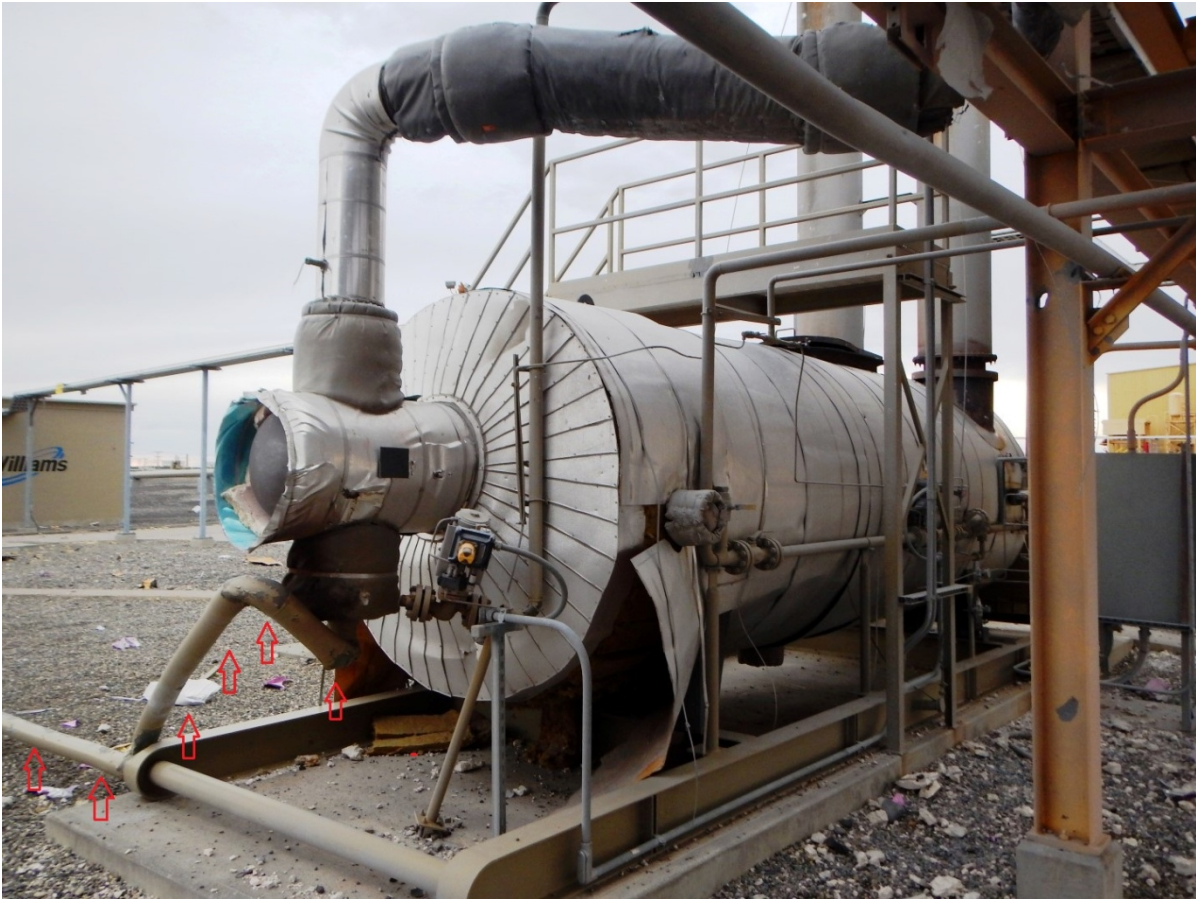
Another view of the Salt Bath Heater. The 4-inch gas inlet piping denoted with red arrows. The piping is blown to the left of the heater. Looking northwest.
