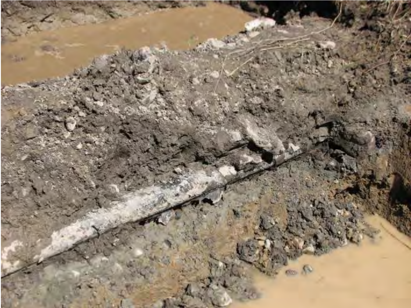
PHOTO 6: ROCKY SOIL AROUND PIPE UPSTREAM DIG 8/29/10
