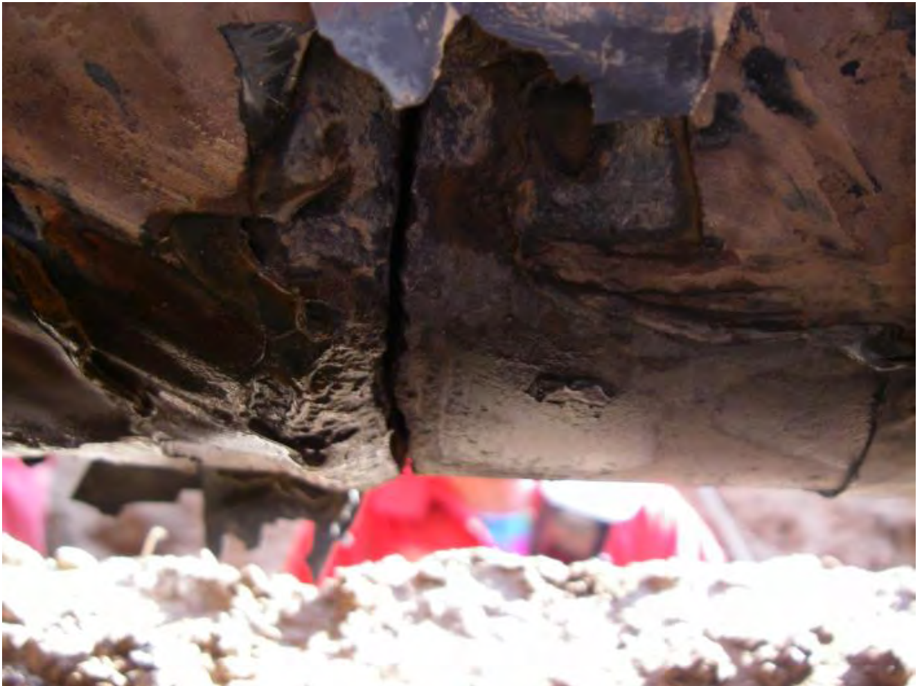
PHOTO 22: CRACK PARTIALLY EXPOSED 09/01/10
