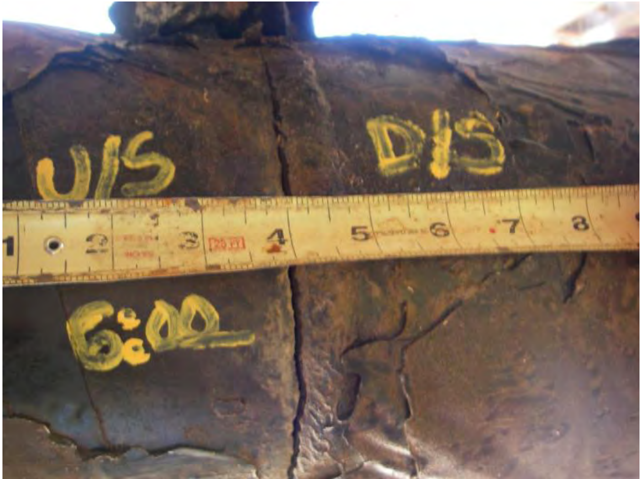
PHOTO 23: CRACK ON BOTTOM QUADRANT'S OF PIPE 09/02/10
