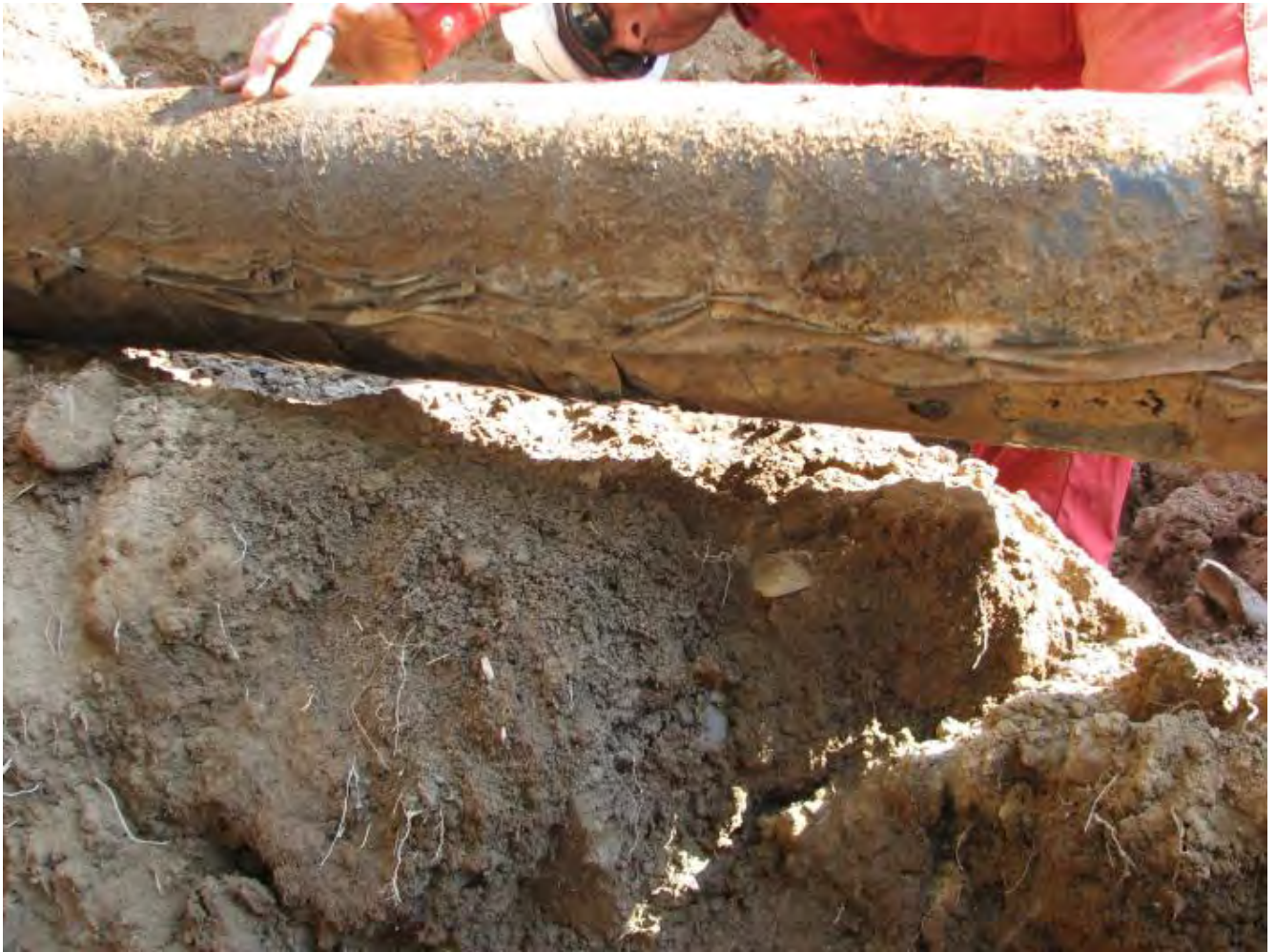
PHOTO 21: EXAMINING PIPE IN AREA OF SUSPECTED LEAK 09/01/10
