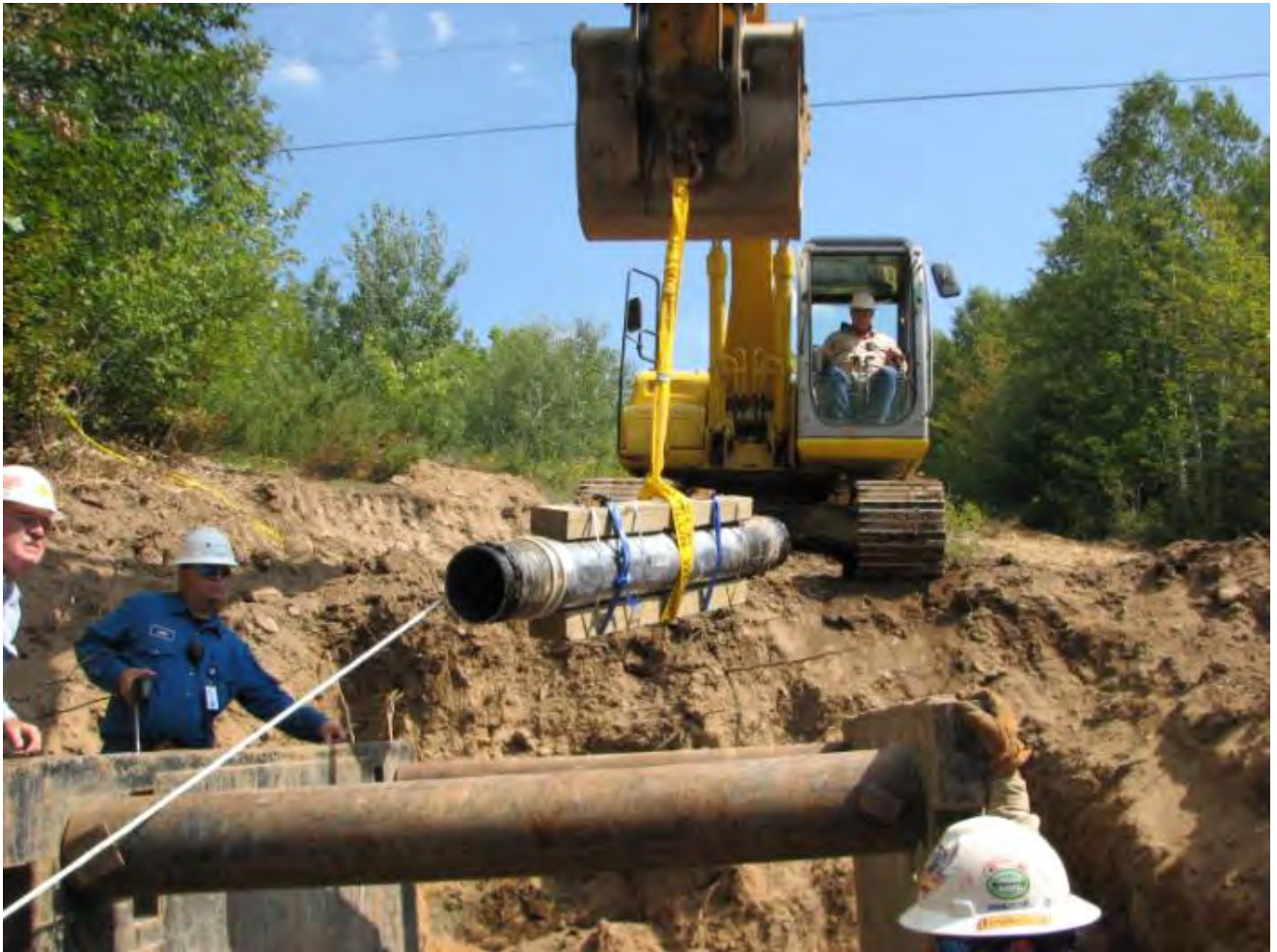
PHOTO 25: PIPE SPECIMEN REMOVED 09/02/10
