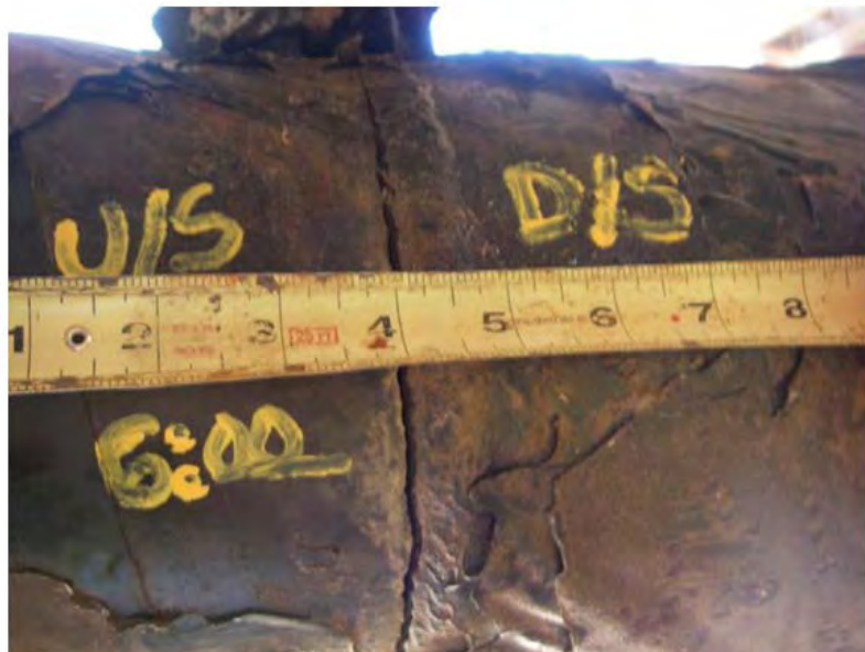
Crack on bottom quadrant of pipe – 09/02/2011
