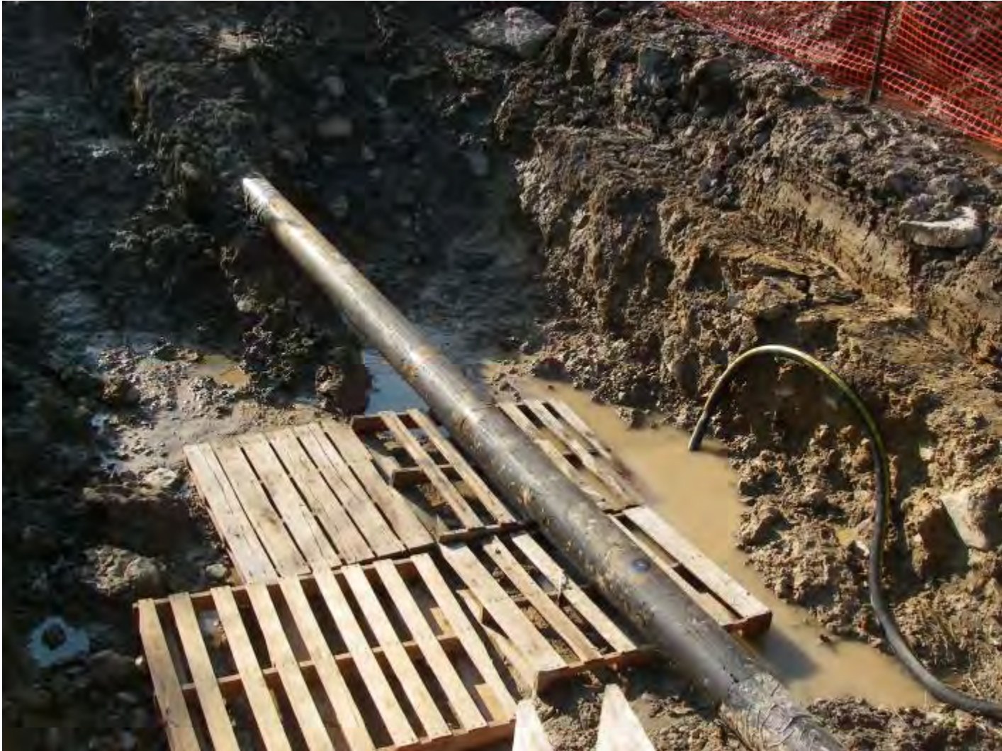
PHOTO 11: EXPOSED PIPE UPSTREAM DIG 8/30/10
