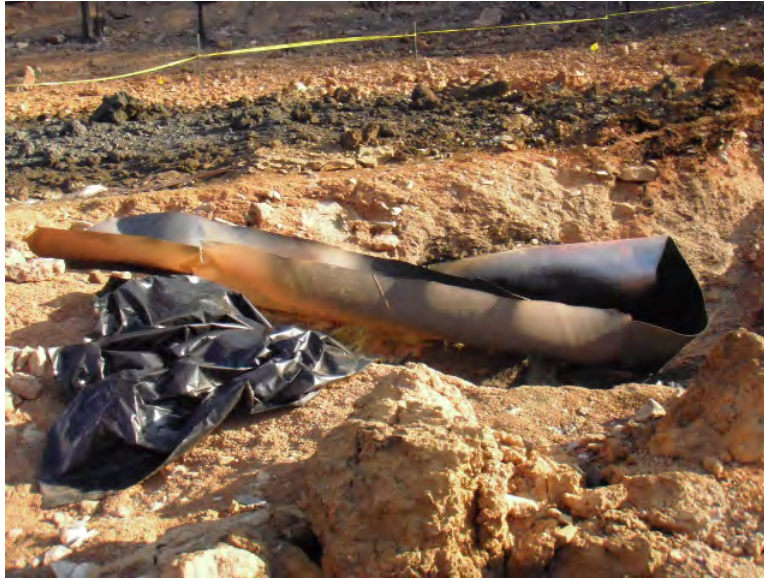
Figure 7. Downstream terminus – High Energy Rupture
