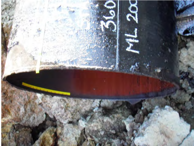
Figure 11. Clean fracture in the girth weld at the upstream pipe terminus – this was location of the Low Energy Failure origin
