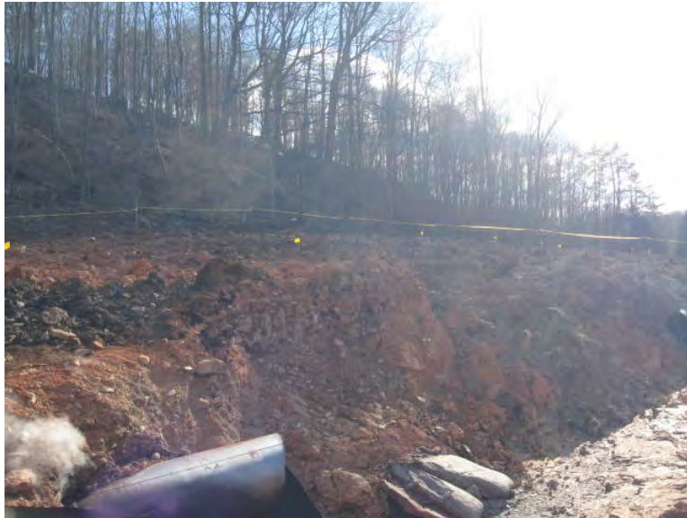
Figure 6. Bottom left of photograph is downstream pipeline failure terminus. The middle/far right of photograph is the upstream pipeline failure terminus
