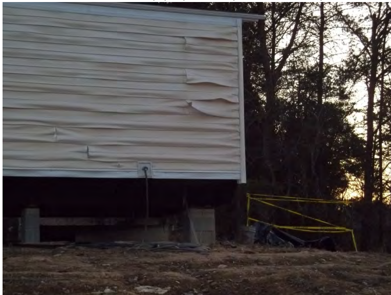
Figure 13. Closer view of heat damage – the yellow tape indicates the location of Line 200 pipe piece expelled from rupture area
