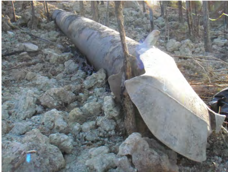
Figure 10. Low Energy Failure pipe section – fractured pipe portion shown mates to the High Energy Rupture section
