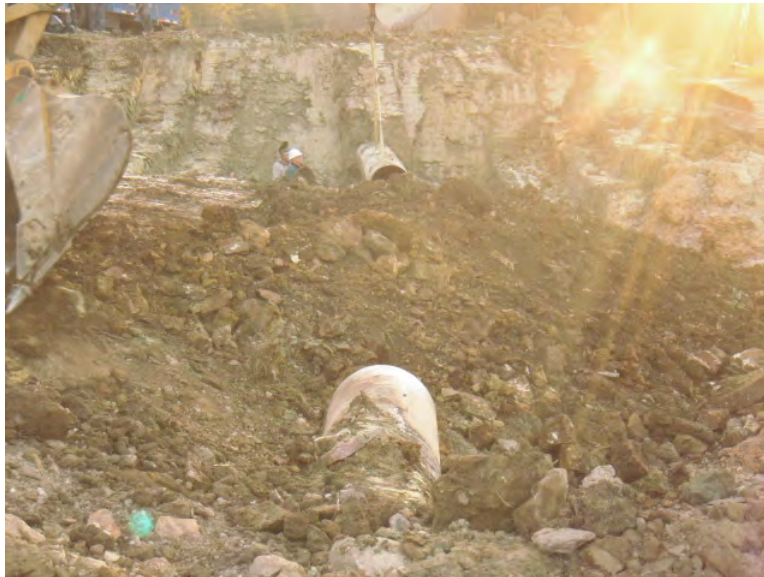
Figure 12. Line 200 looking downstream – The offset between the upstream and downstream termini necessitated the over bend and side bend during the original construction
