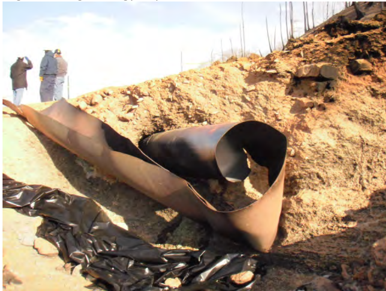
Figure 8. High Energy Rupture section
