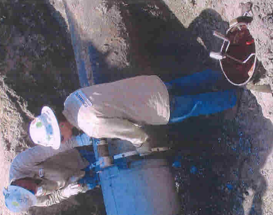
Williams-Transco 24-inch "A" Pipeline King Ranch MP 97.53, 04-28-2010 Cold-Cutting 24-inch Pipe Note: Bonding Cable Attached to Equalize Electrical Potentials on Each Side of Cut
