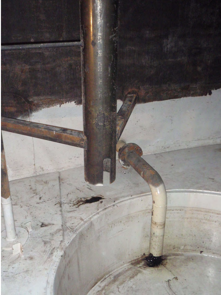
Water draw sump inside the tank. Gauge tube can be seen.
