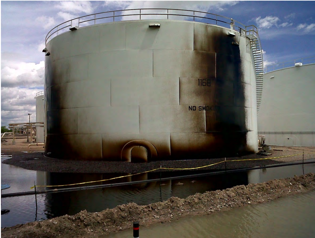
Suncor Tank 1168 Overfill.
