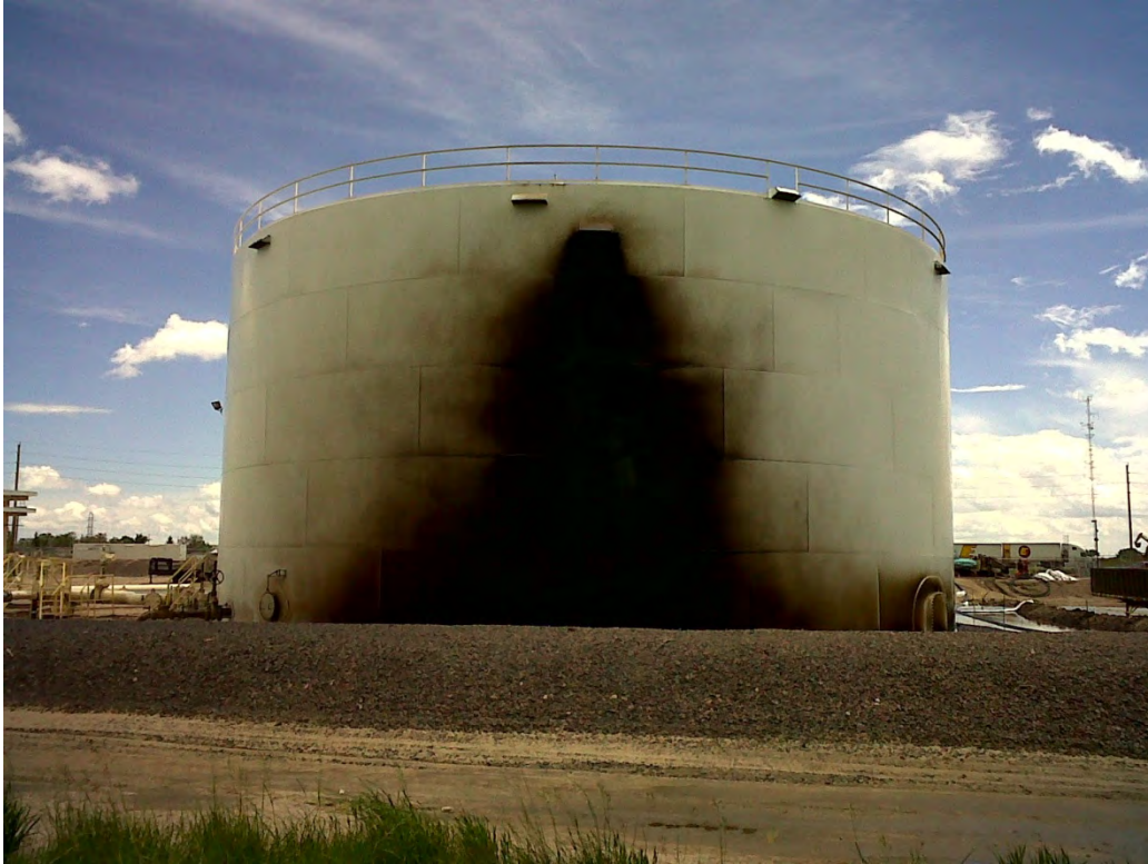
Suncor Tank 1168 Overfill.
