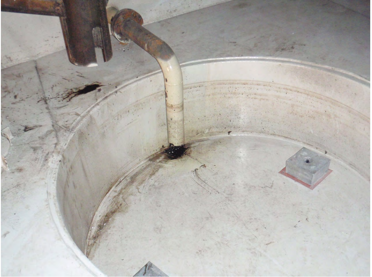
Water draw sump inside the tank. Gauge tube can be seen.
