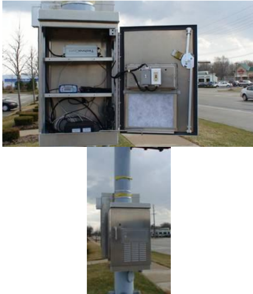
Figure 8: CICAS-V Intersection Equipment
