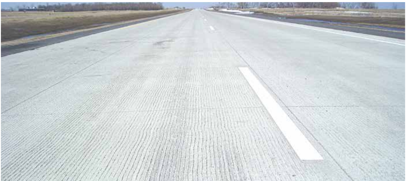
This finished 7-inch whitetopping surface with pavement marking was completed as part of an FHWA Highways for LIFE supported pavement rehabilitation with North Dakota DOT. (Image source: FHWA)
