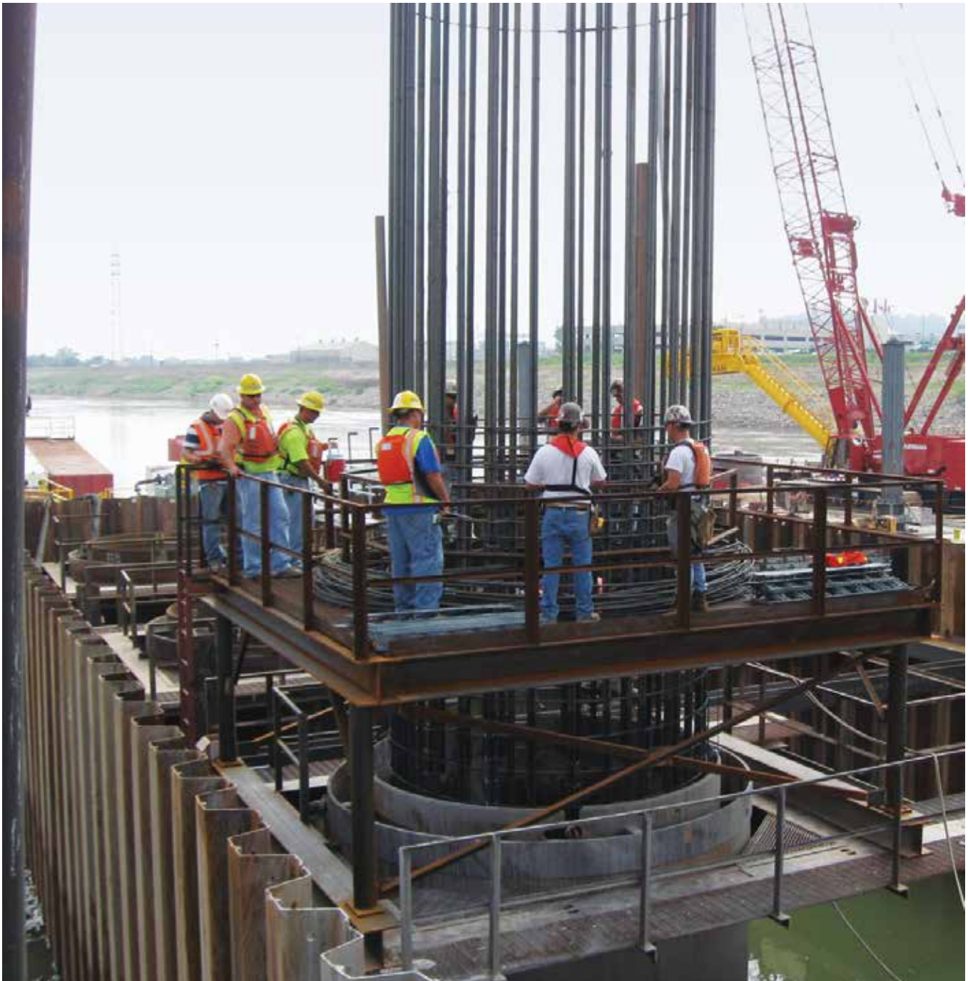
FHWA's Highways for LIFE program supported the Missouri DOT's construction of the Christopher Bond Bridge through an innovative design build procurement process. The bridge foundations were designed and constructed using cost-effective technical engineering solutions that led to significant savings in time and money. (Image source: FHWA)
