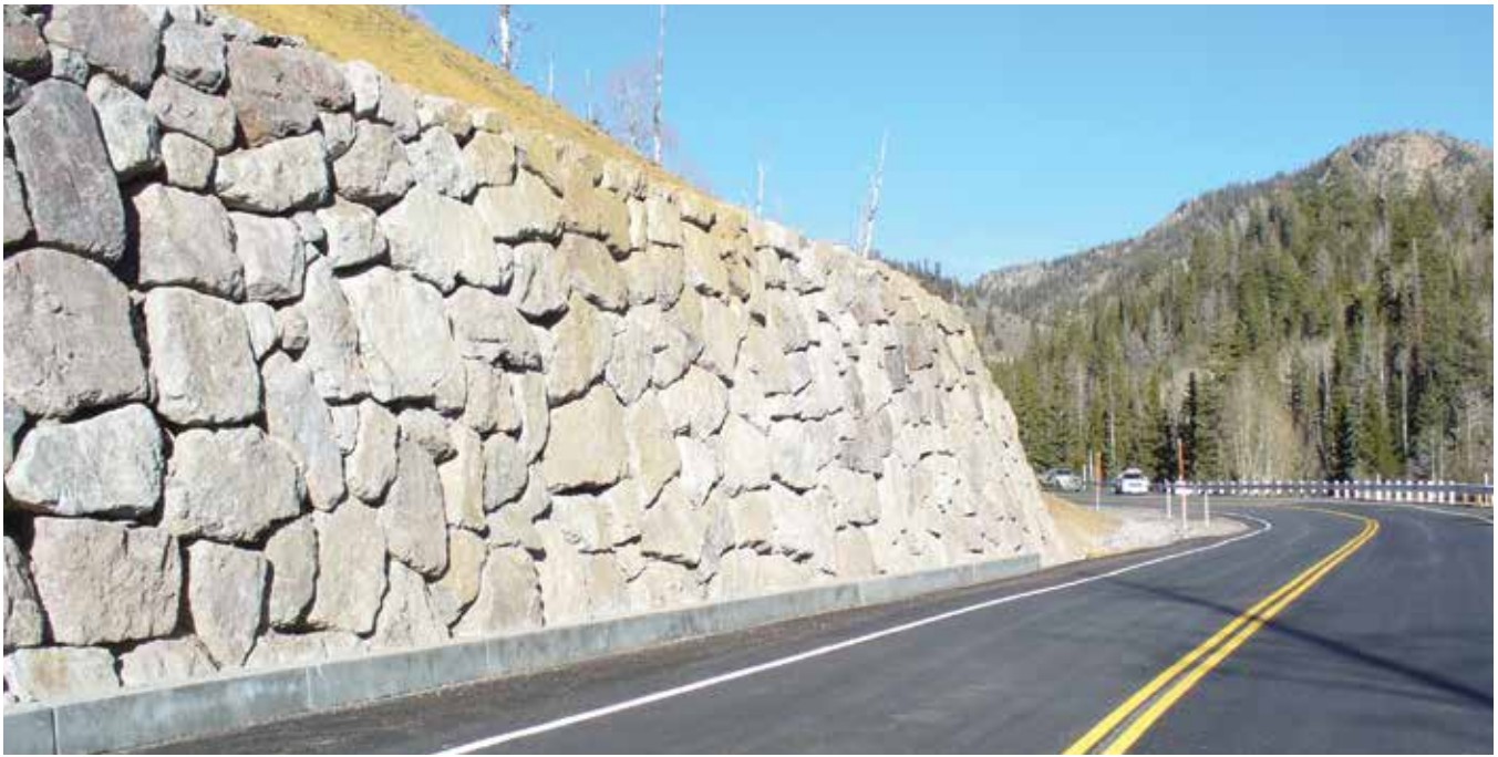
FHWA guidelines on building rockeries, like this one on State Route 153 in Utah's Fishlake National Forest, have reduced the cost of building walls by as much as 50 percent. (Image source: FHWA)
