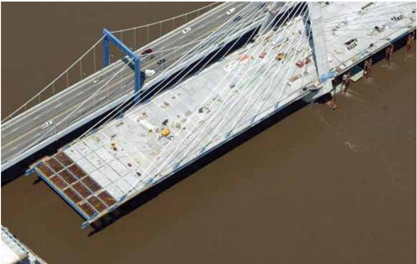
Construction of the roadway surface nears completion on the Christopher Bond Bridge construction project in Kansas City, Missouri. The innovative side-by-side bridge construction technique saved time and minimized road closures. (Image source: FHWA)
