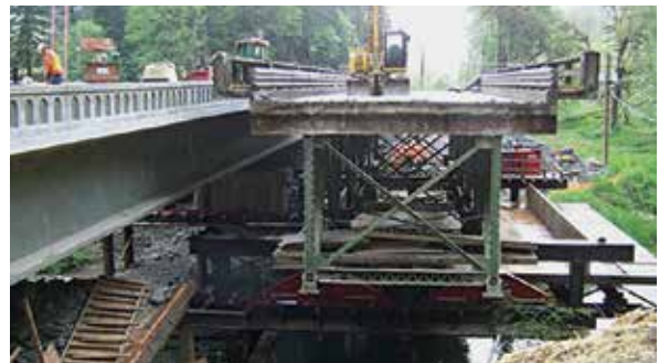
Top: Trucks deliver concrete for the deck of the existing Paseo Bridge in Missouri as part of a project that used innovative design techniques to accelerate bridge construction. Above: FHWA and Oregon DOT use accelerated bridge construction to rapidly remove and replace five bridges on Oregon 38. Rapid bridge replacement technology used hydraulic jacks mounted on a sliding rail to slide the old superstructure onto temporary supports and move the new superstructures into their final position. (Images: FHWA)
