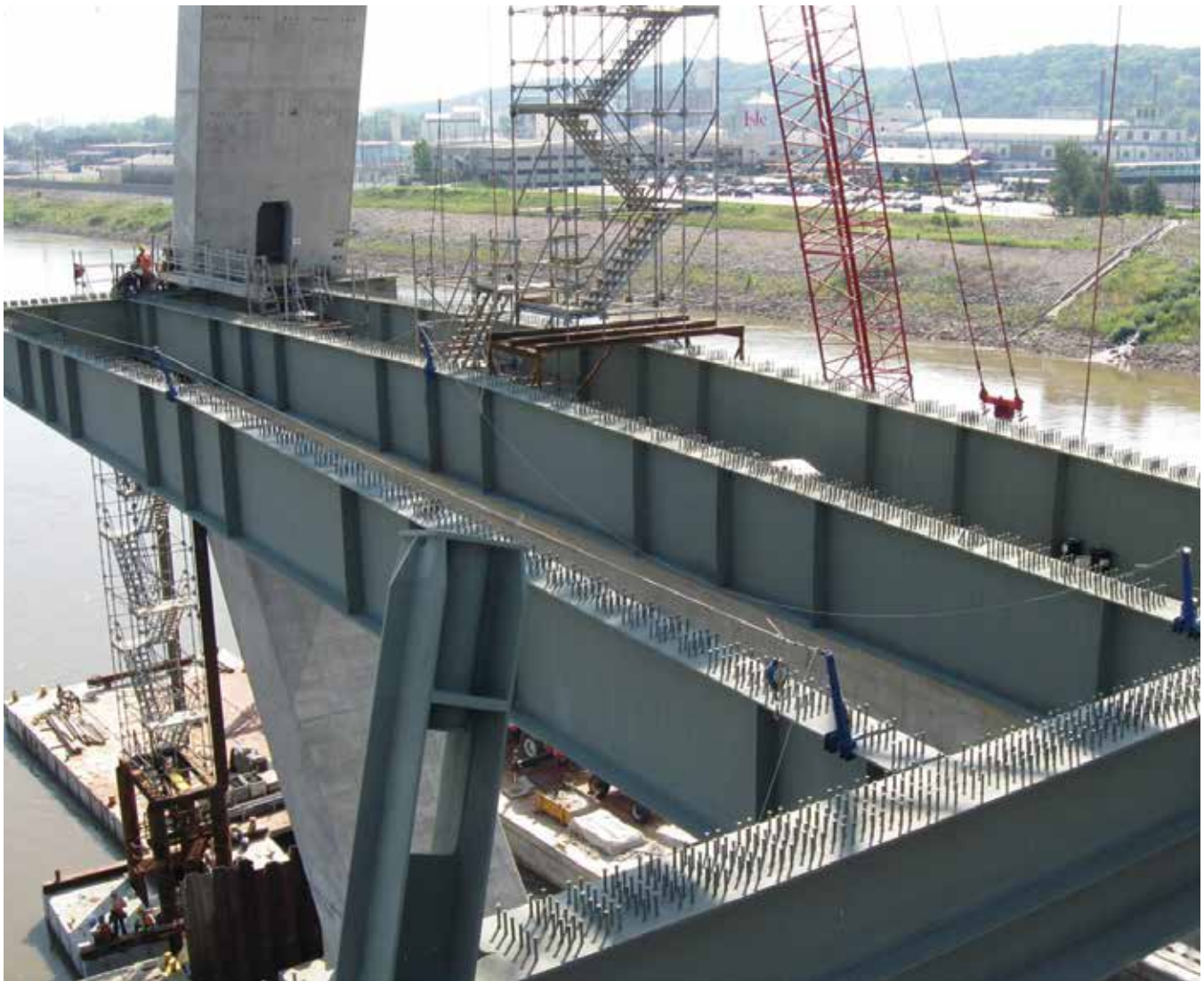
FHWA's Highways for LIFE program supported the placement of the pier table on the deck of the Christopher Bond Bridge through an innovative design build procurement process, providing cost savings and flexibility in the bridge construction schedule. (Image source: FHWA)
