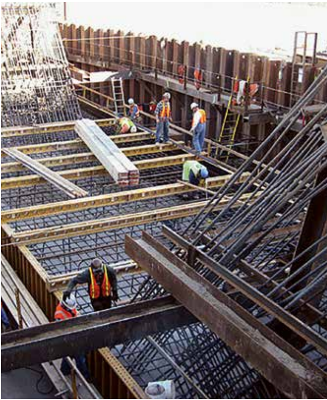
Placing of rebar prior to concrete pour during construction of a pylon on Christopher Bond Bridge construction project was one of many cost-effective, technical engineering solutions that saved time and provided flexibility in the bridge construction schedule. (Image source: FHWA)
