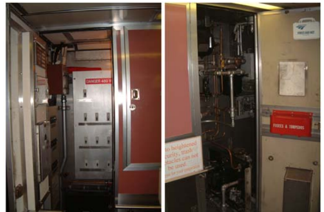
Figure 9. Electrical and Brake Service Closets, MBTA Commuter Car, built by Kawasaki
