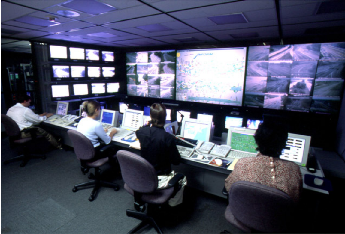
Figure 4-1 INFORM (Long Island, NY) control center.
