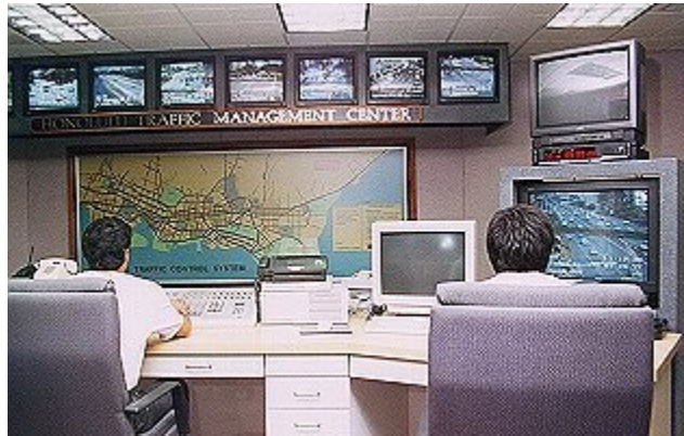
Figure 8-1 Traffic management center (TMC) (1).
