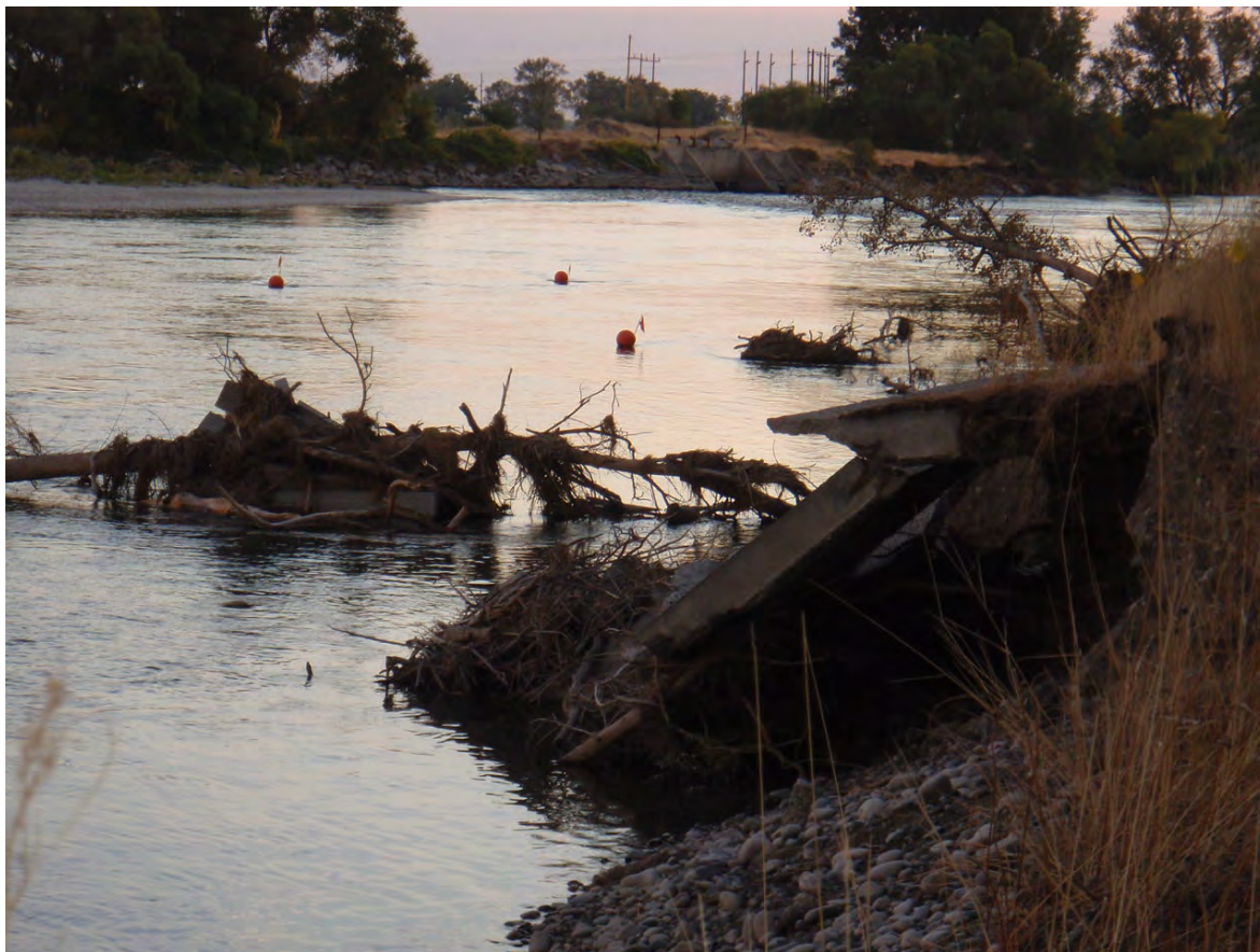
Looking NE from south bank of the Yellowstone River at the boat ramp just upstream of the EMCO crossing. Picture was taken Thursday, September 29, 2011, 2:52:11 PM after the river level dropped. One can see the same debris pile in the river as was in the last picture. The concrete seen in the foreground of this picture is the boat ramp in the previous picture. The buoy furthest to the right is marking the north end of the rupture from the south bank. The next buoy is marking the south end of the rupture from the north side of the main channel off of the island.
