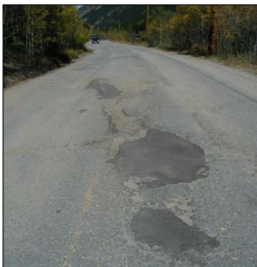
Figure I-3 Distressed Pavement Conditions
