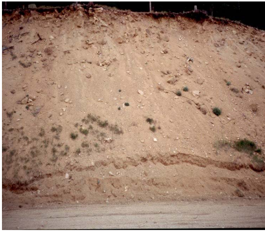
Figure III-5a: Unvegetated, unstable cut slope with toe of slope undercut.
