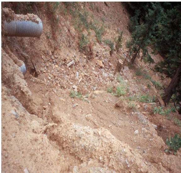
Figure III-5c: Sediment discharge from a 'hanging' culvert erodes a slope and deters vegetation growth.
