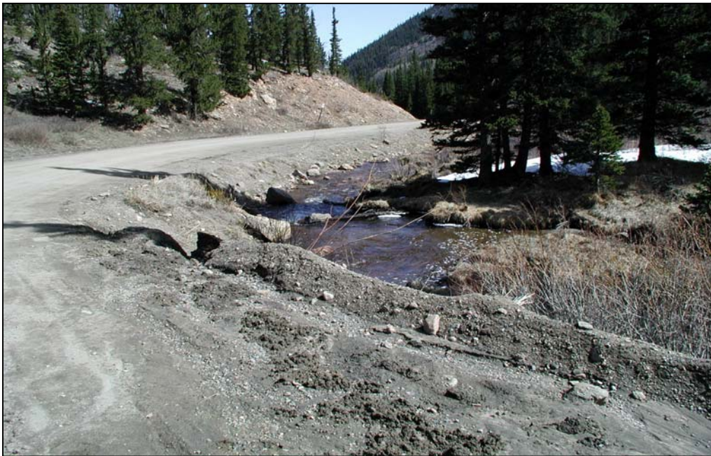
Figure I-10 Spreading and erosion of road materials into sensitive habitats
