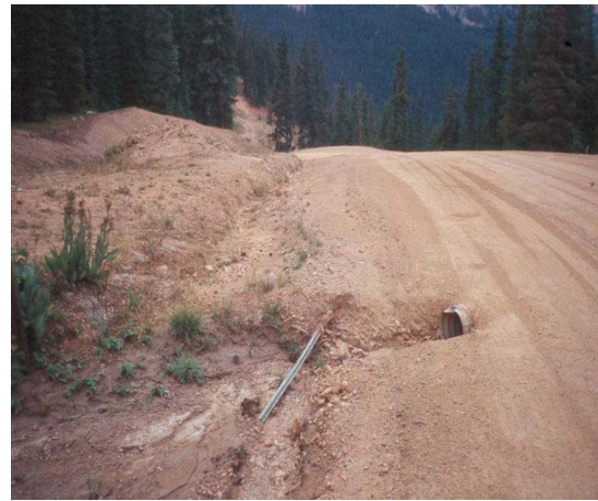
Figure III-5b: Roadway maintenance has pushed the road beyond its original boundaries.
