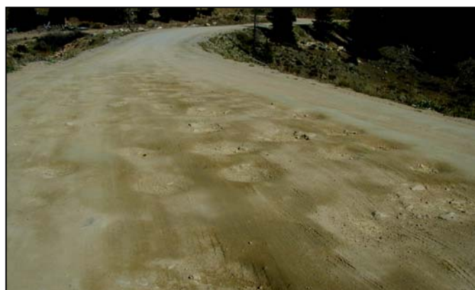
Figure I-4 Pot-holes and Ruts on a Gravel Section
