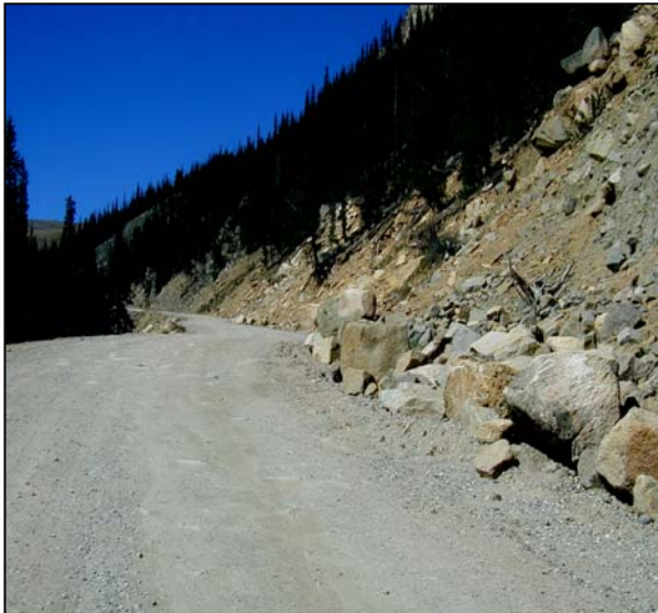
Figure I-8 Steep Cut Slopes and Heavy Rockfall
