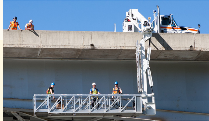
Pictured are researchers, contractors, and Alaska DOT&PF staff installing a fiber-optic remote structural health monitoring system on Alaska's Chulitna River Bridge. (Source: M. Fisher)
