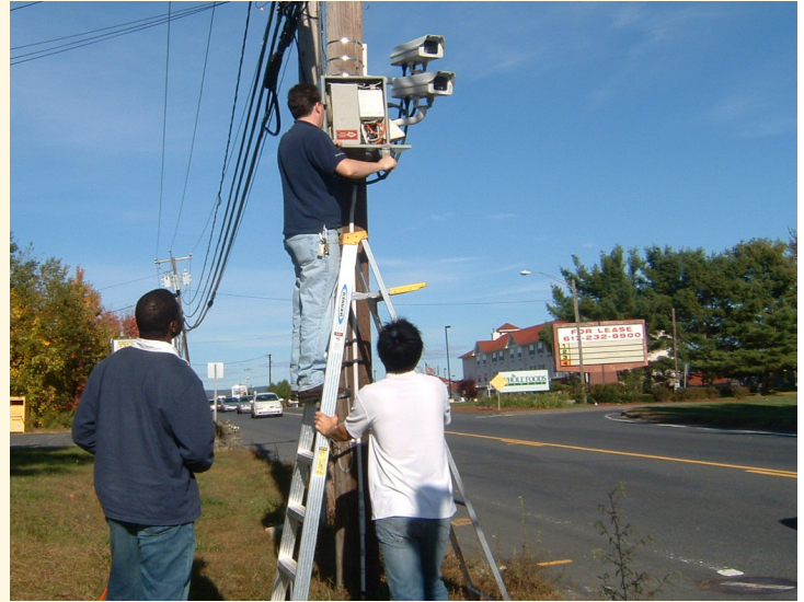
James Schleicher, RTIC Systems Engineer along with two UMass students (Dwayne Henclewood, MS 2007 and Haizhong Wang, PhD 2010) install traffic sensors in the field. Photo courtesy of Dr. Daiheng Ni, Associate Professor, Civil & Environmental Engineering at UMass Amherst.
