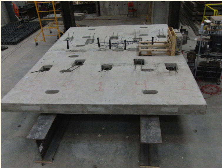
Layout of full-scale precast concrete deck panel specimen prior to grouting. Photo courtesy of UTC.
