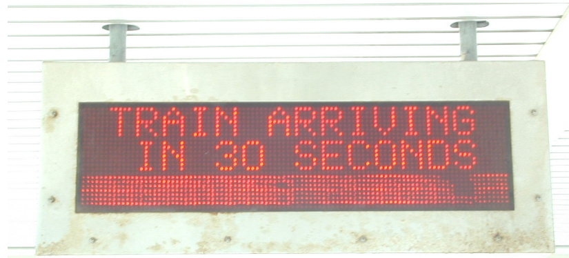
Figure 3-8. Jacksonville Transportation Authority's PIDS
