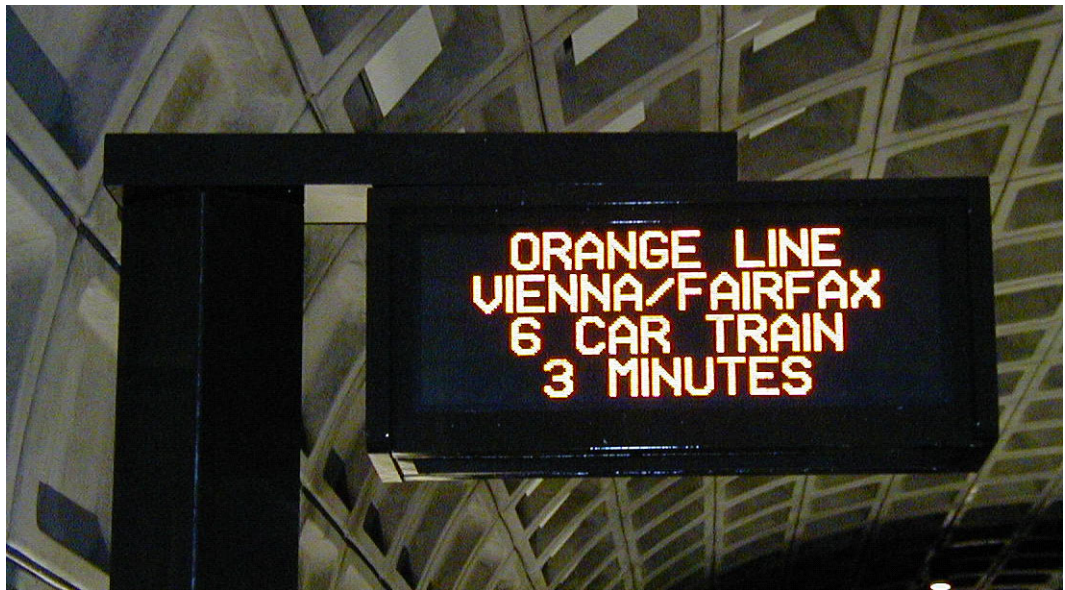
Figure 3-2. Washington Metropolitan Area Transit Authority LED Passenger Information Display
