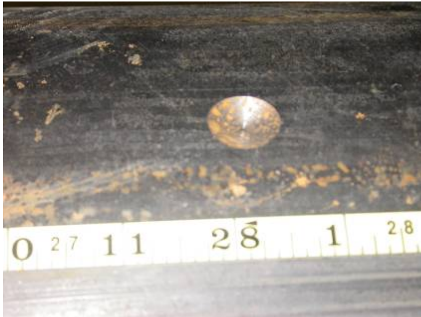
Figure 2-34. Defect P3-9 (Defect 6)
