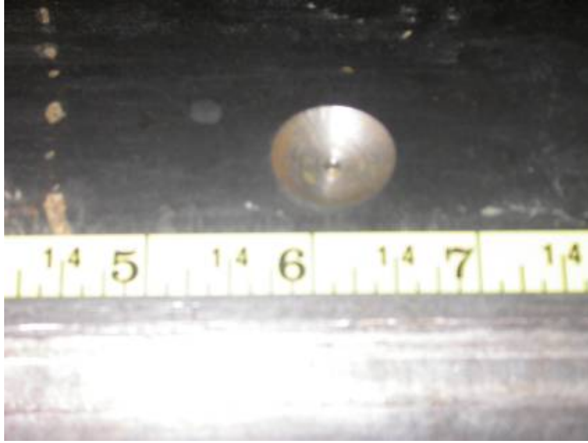
Figure 2-31. Defect P3-4 (Defect 3)
