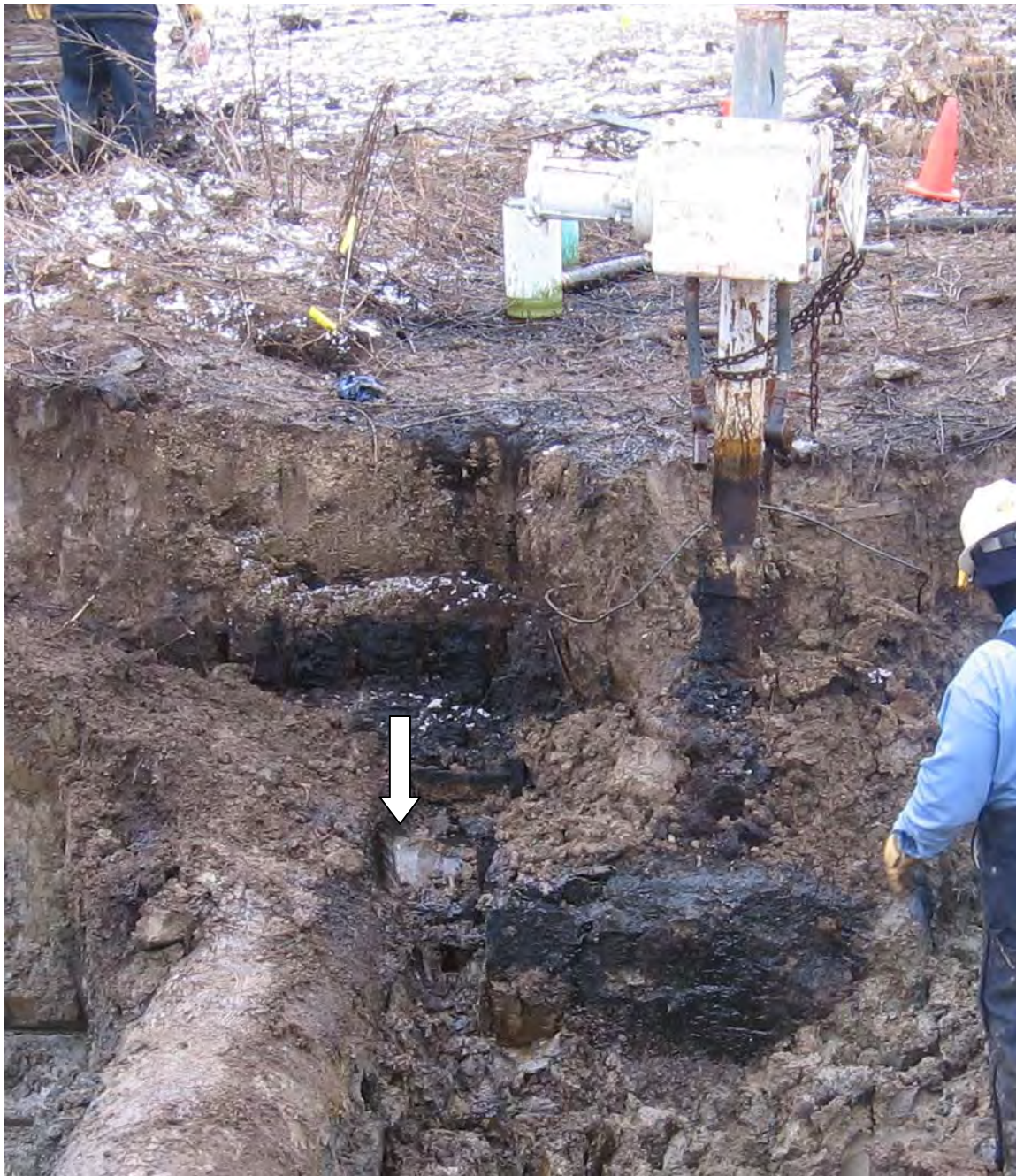
Photo 6 - The photo shows origin of the leak. The arrow points to the crack.
