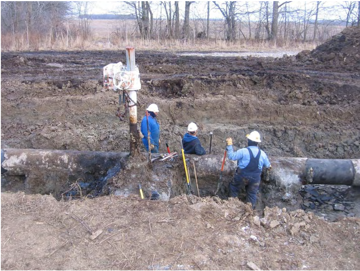
Photo 4 - The photo shows the valve actuator at the branch connection.
