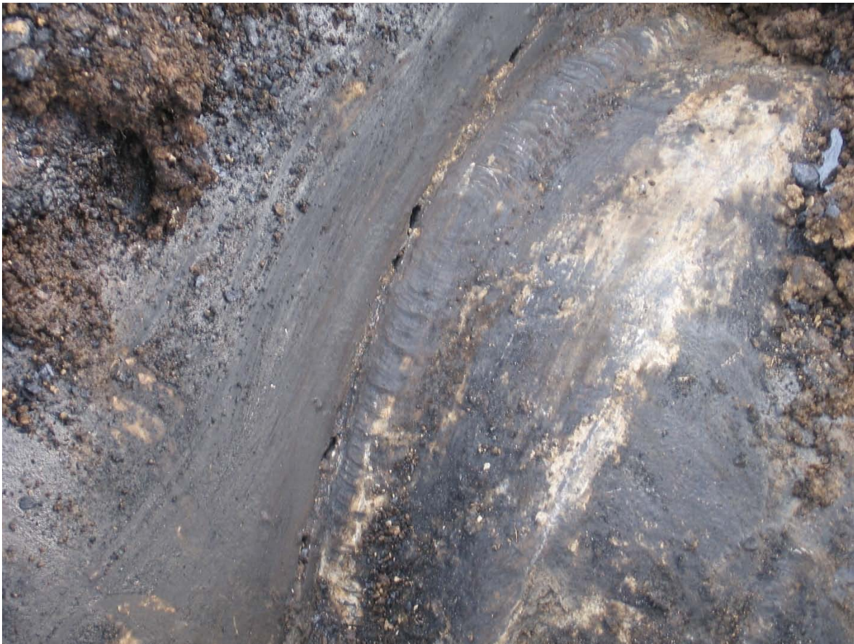
Photo 8 - The photo shows the crack. Note the crack does contain some dirt as the result of the excavation.
