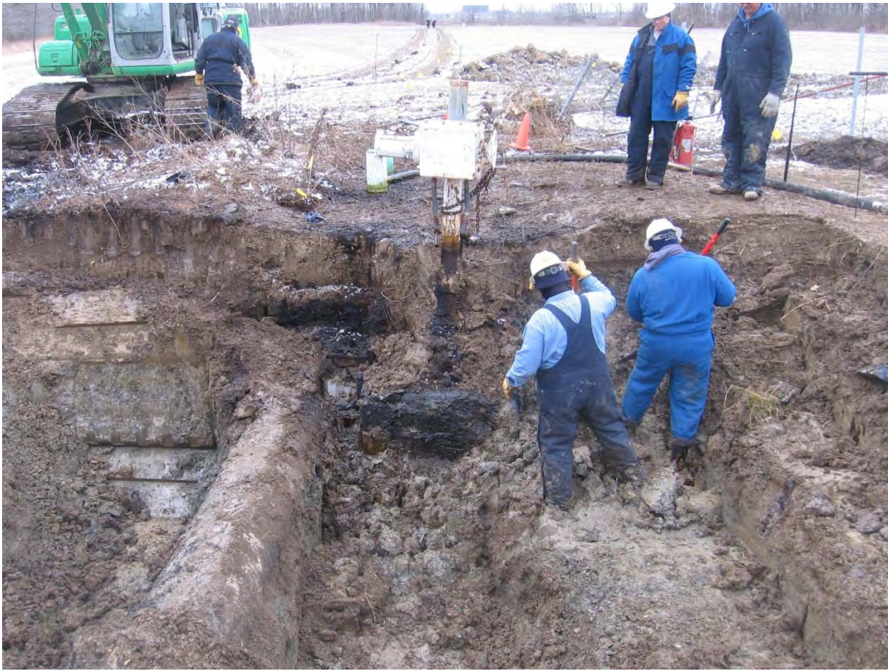
Photo 2 – View from leak site looking south. Visible is the branch connection and 12" valve.
