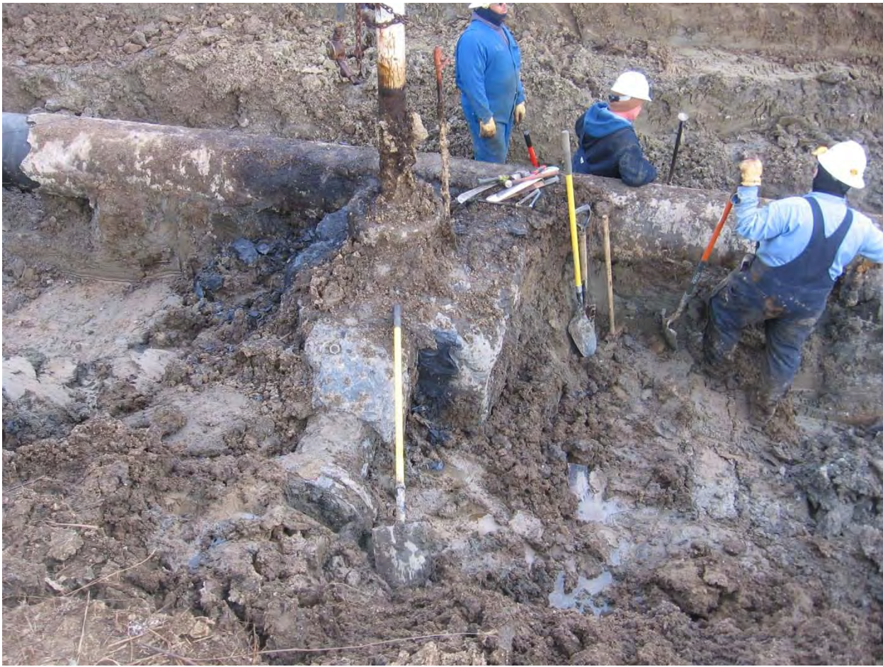
Photo 5 - The photo shows the valve and blinded flange.
