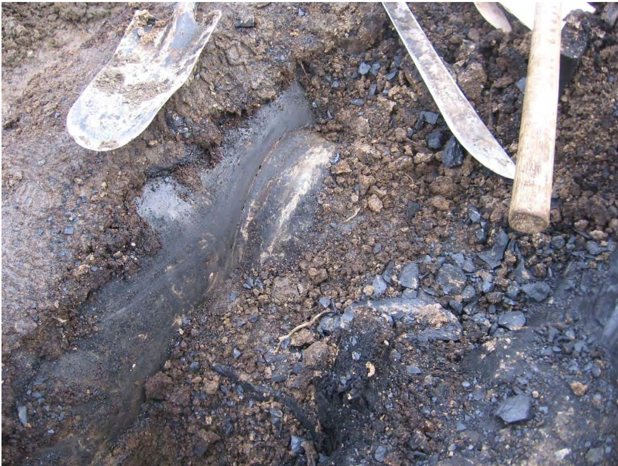
Photo 7 - The photo shows the weld between the mainline pipe and the branch connection.
