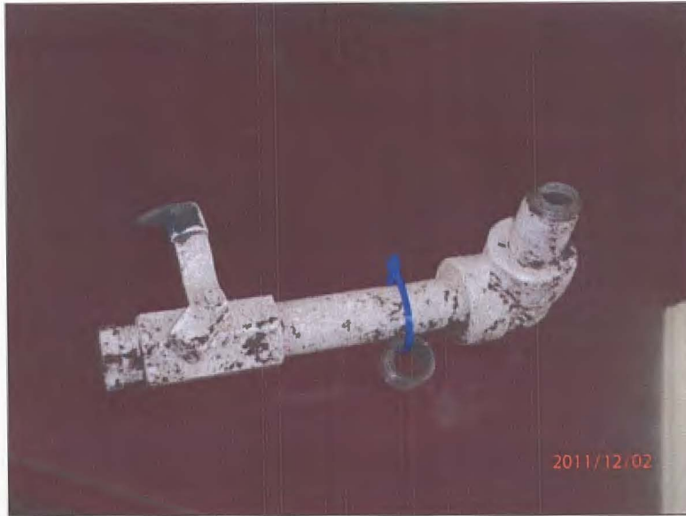
Picture 6 - Drain line that was damaged
