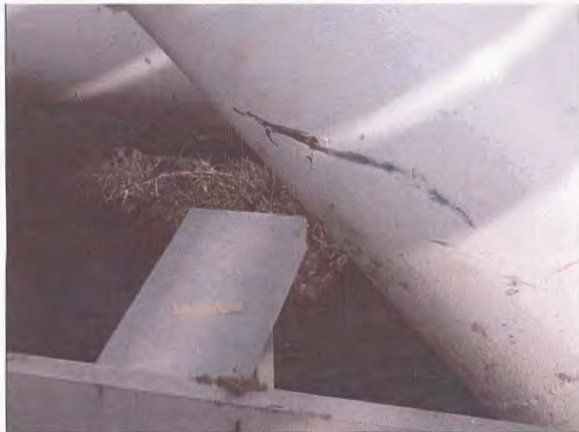
Picture 5 – Tank Line 3012 showing where it might have hit pipe support
