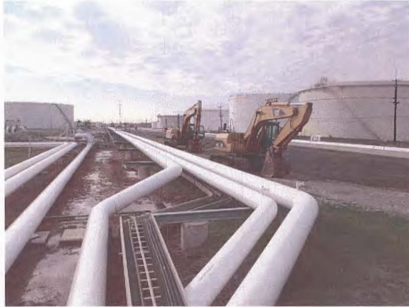
Picture 2 - 20-inch Tank 3012 Pipeline – looking towards Tank 3012
